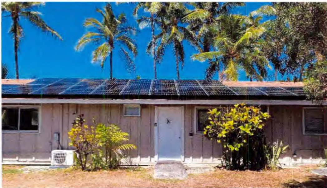
Figure 5.3.5. PV system installed on the MMRP building.
