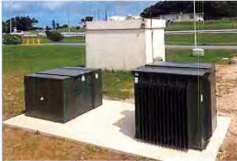
Figure 5.2.4. Installed VR and bypass switch.
