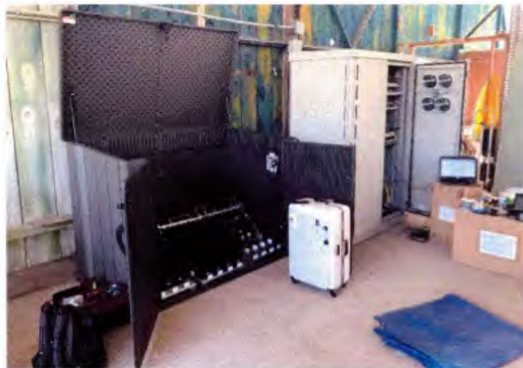
Figure 5.3.2. Swap battery charging station and portable BESS units.
