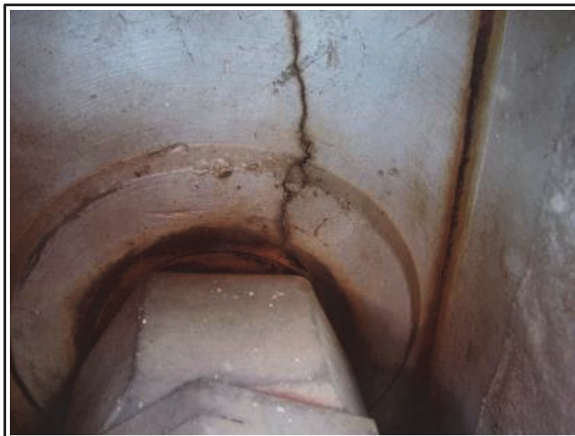
Figure 33. Crack caused by flushing accident at Lockport Lock.
