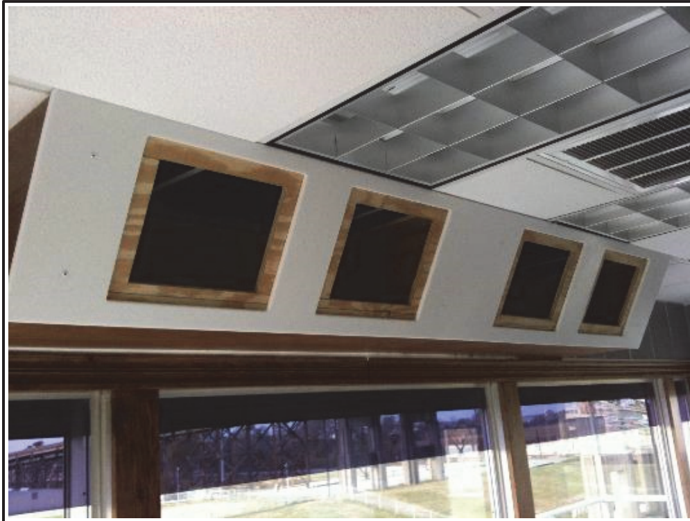
Figure 11. Overhead monitors control room Port Allen.
