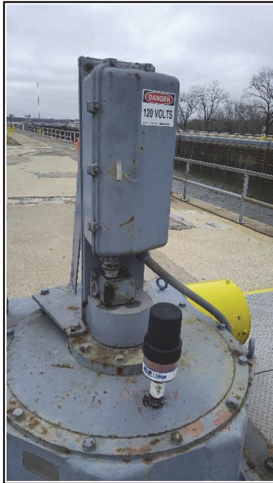
Figure 9. Old cam-operated limit switch gearbox at Brandon Road Lock.
