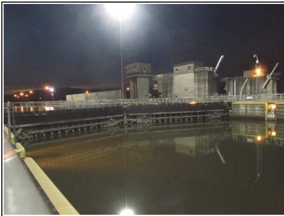
Figure 39. High mast LED lighting at Winfield Locks and Dam.
