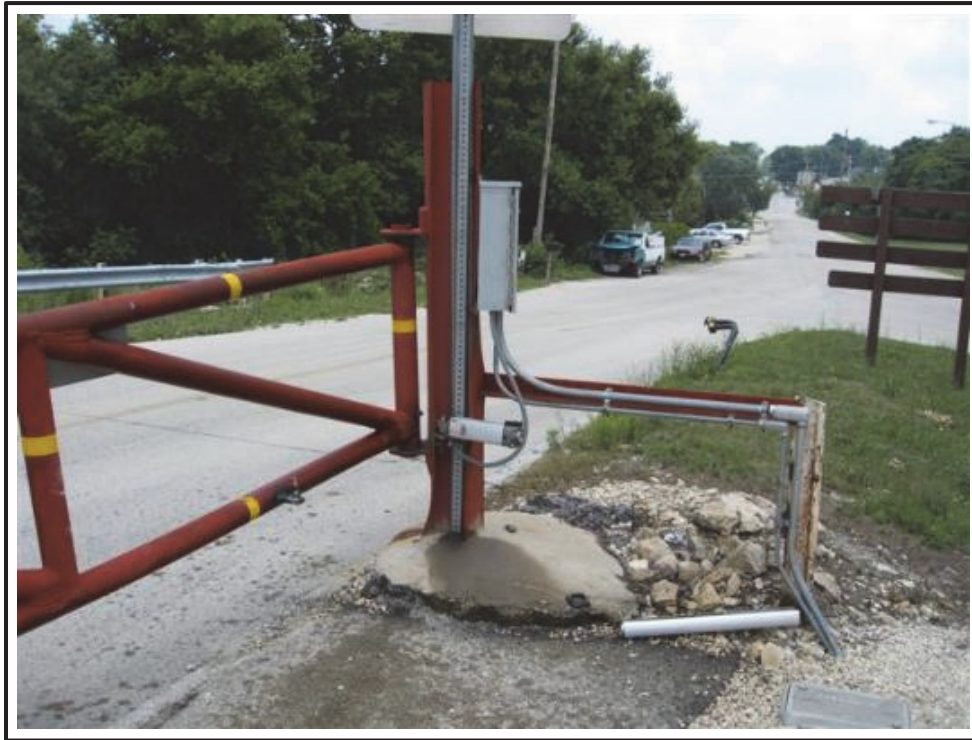
Figure 37. Bridge security gate damage at 16 th Street.
