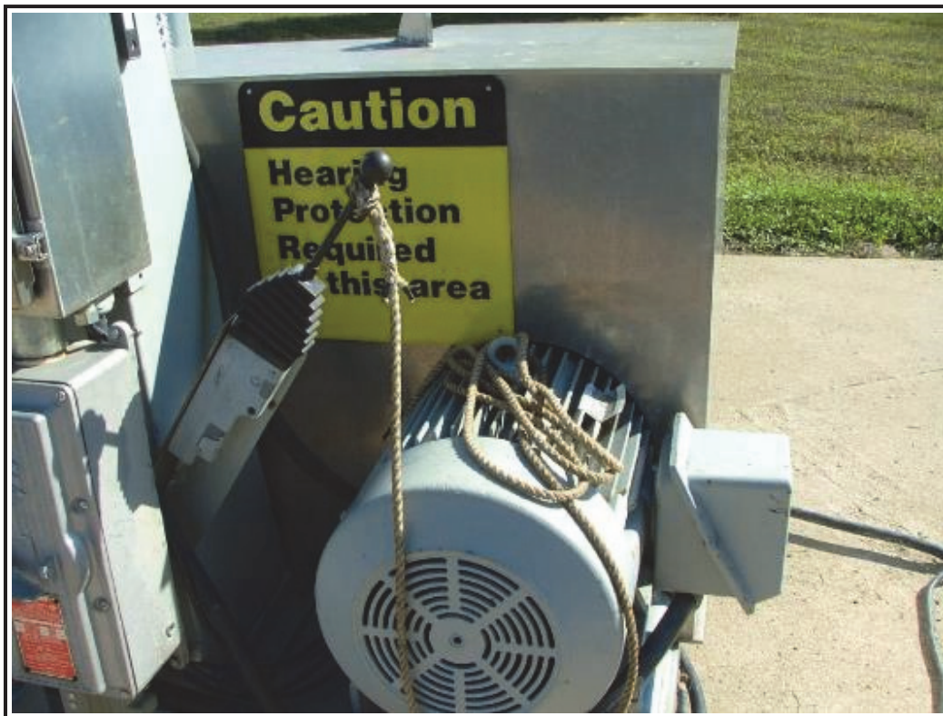
Figure 35. Hydraulic tow haulage unit at Peoria Lock.
