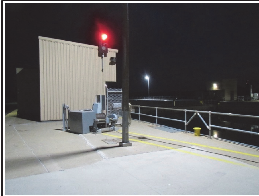
Figure 44. Tow haulage unit lighting at Lockport Lock.
