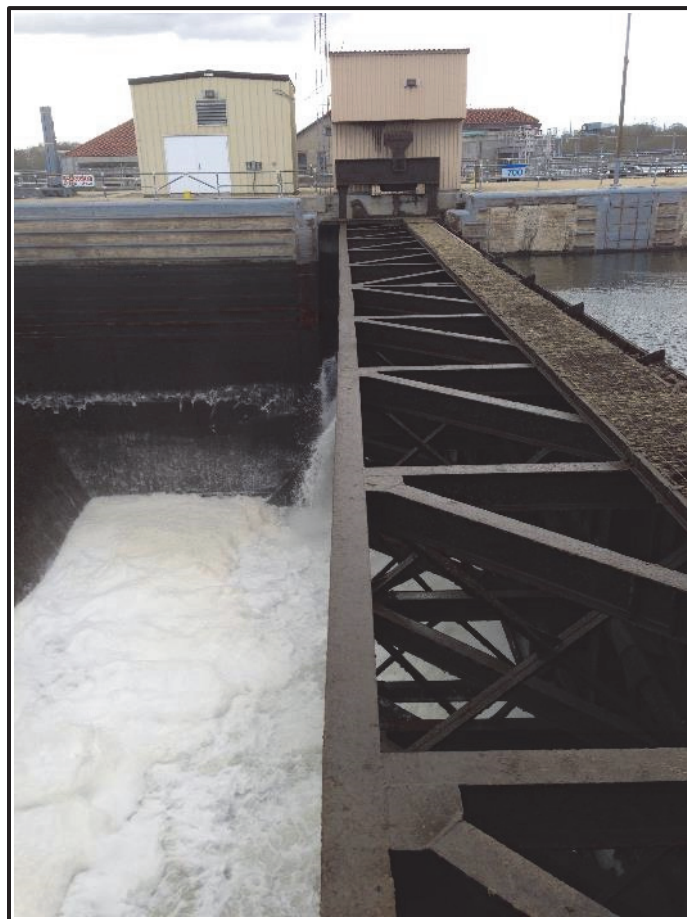
Figure 34. Lockport Lock emergency gate bent beam damage.
