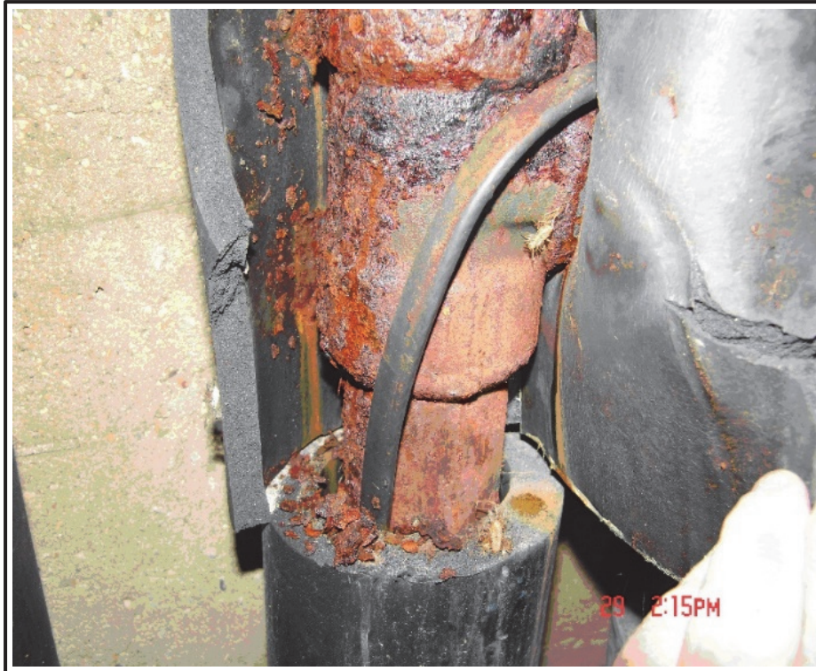
Figure 23. Hydraulic system on emergency gate.
