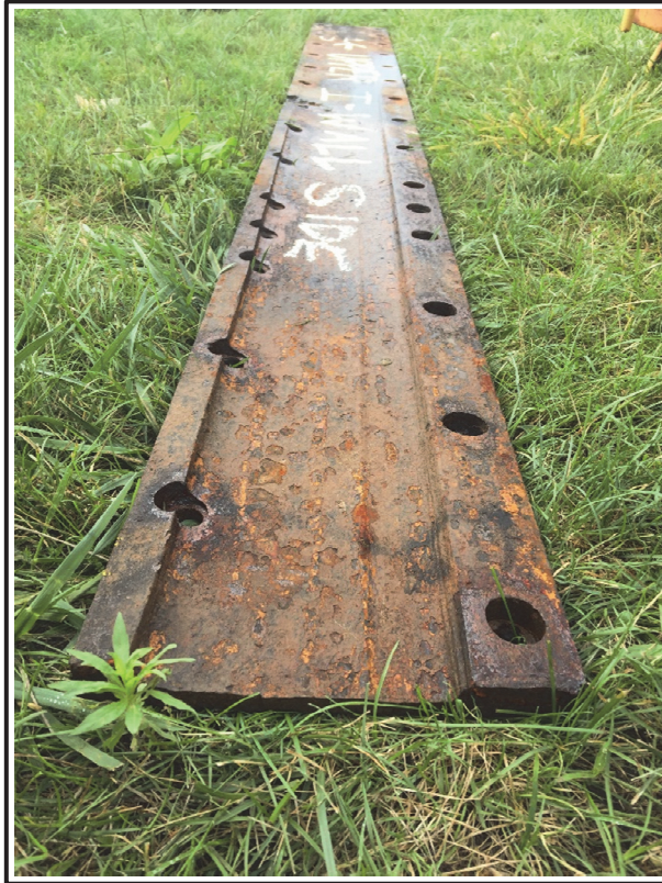
Figure 22. Lower valve wear tracks at Lockport Lock.
