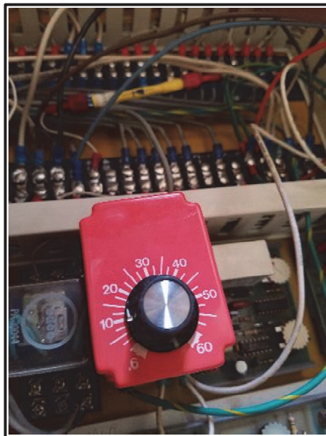
Figure 38. Generator solid-state time-delay relay at Lockport Lock.
