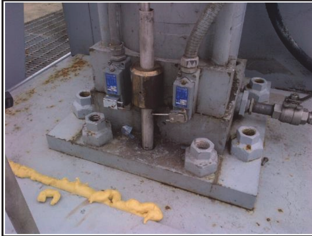
Figure 7. Close-up of redundant closed switch at Starved Rock Lock.
