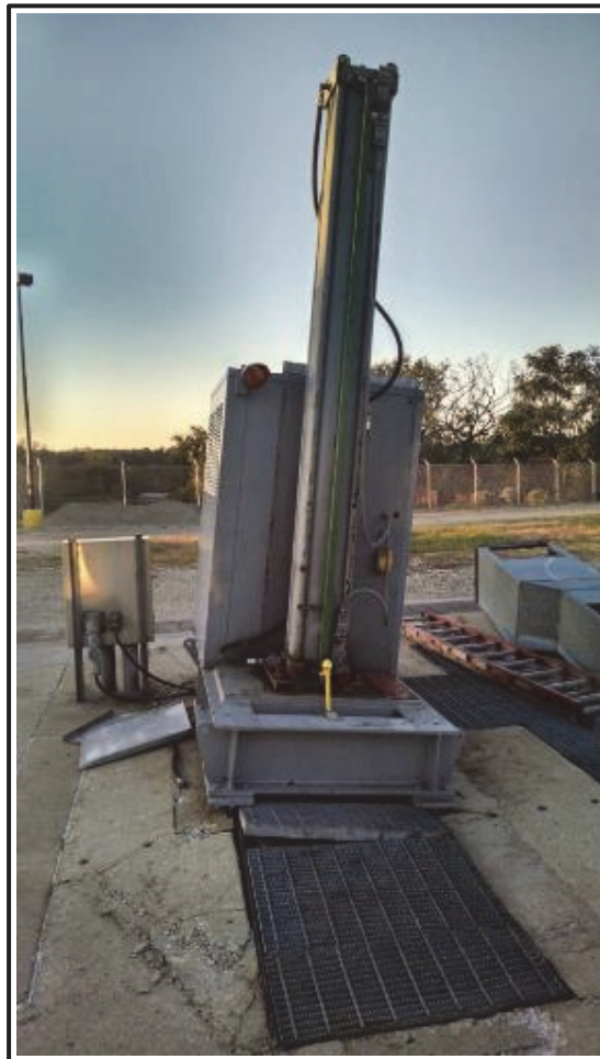
Figure 30. Brandon Road Lock CLOSED limit switch failure.
