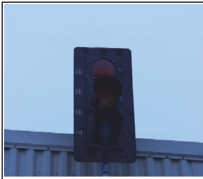
Figure 48. Traditional signal at upstream lock gate.
