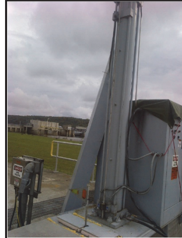
Figure 8. Cam-roller arms on redundant closed switch at Starved Rock Lock.
