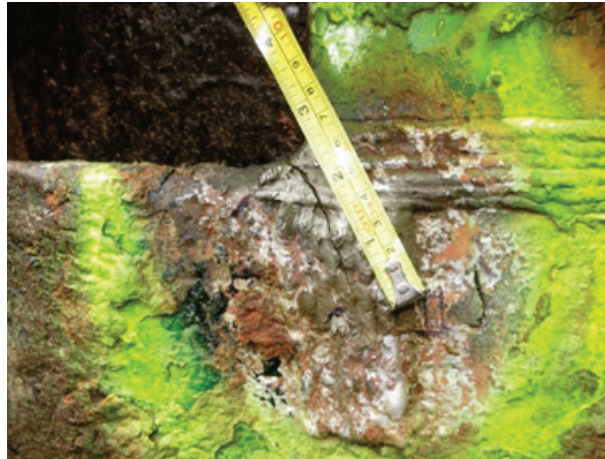
Figure 6. Crack at welded connection (Old Hickory Lock and Dam).
