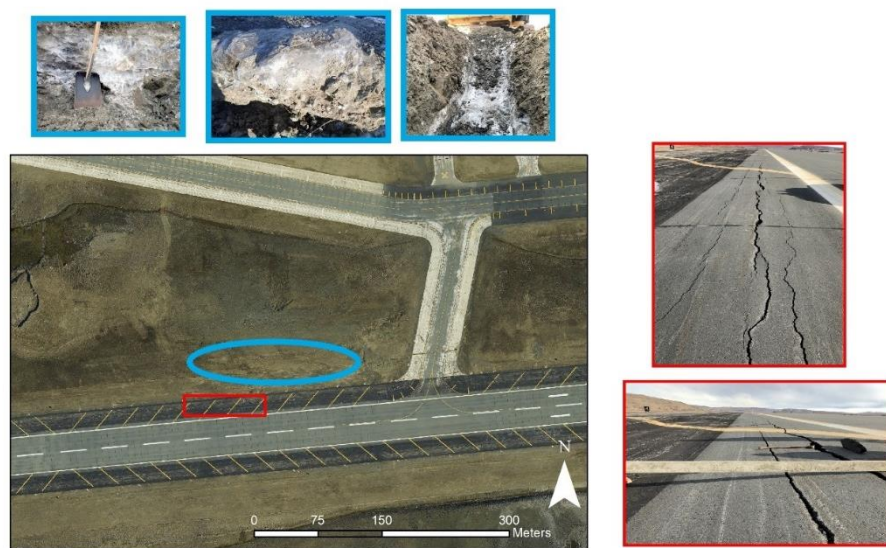
Figure 28. Severe Airfield Damage and Nearby Massive Ice
