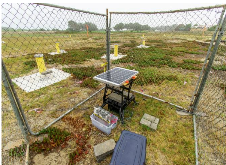
Figure 9. Solar Power Distribution System in Place
