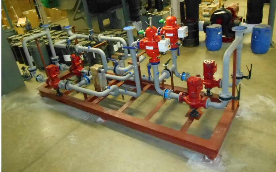
Figure 7. Facilities Liquid Loop Equipment Sled
