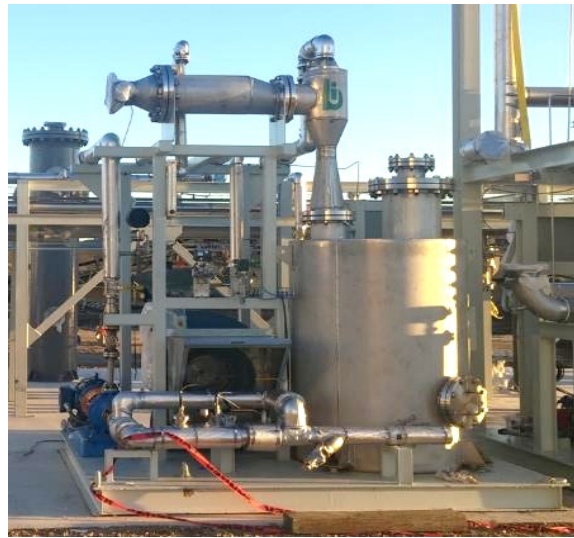
Figure 13. Venturi Scrubber Module at FHL
