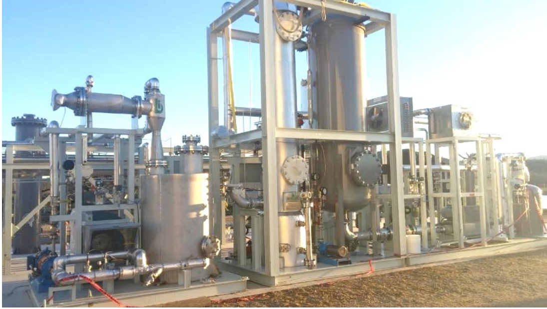
Figure 12. Primary Gas Cleaning Modules at FHL
