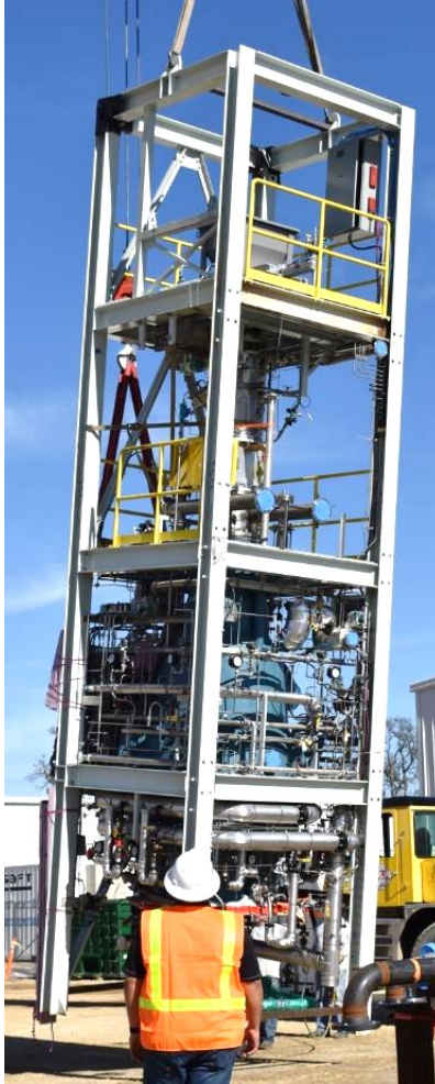
Figure 9. FastOx Gasifier Module Arriving On-site
