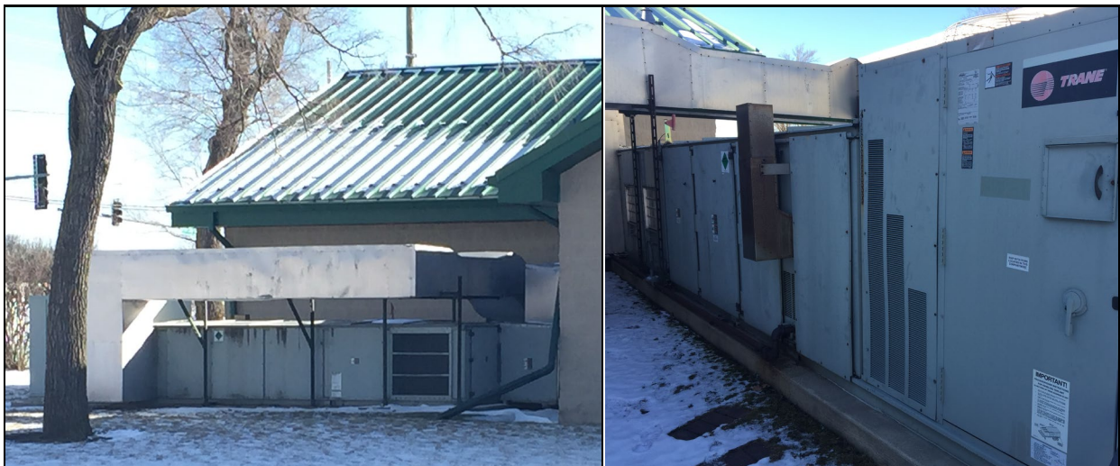
Figure 15. Demonstration Equipment Replaced the Existing Ground-mounted VAV System
