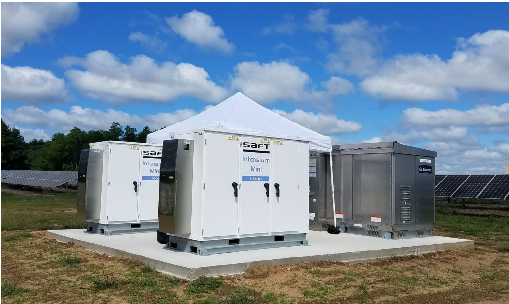
Figure 6. Energy Storage Added to Support Existing PV (in the background)
