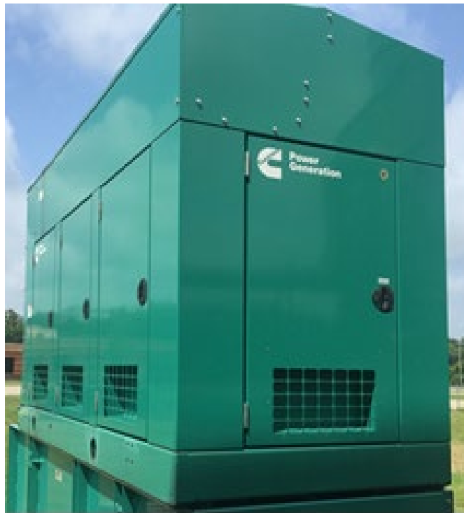
Figure 3. Building 2900 Cummins Generator
