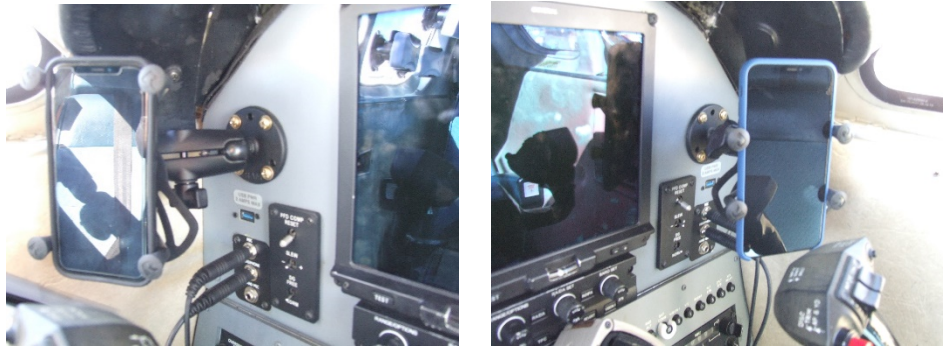
Figure 9: C-12 Cellphone SUT Installation
