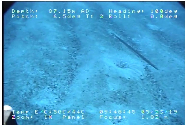
Figure 6: Image captured of the SDL1 (unarmored) cable partially buried in the sand ripples along the submerged shelf. Picture supplied by Sea Engineering, Inc., using their Seamoor Chinook ROV suspended from the workboat Huki Pono .
