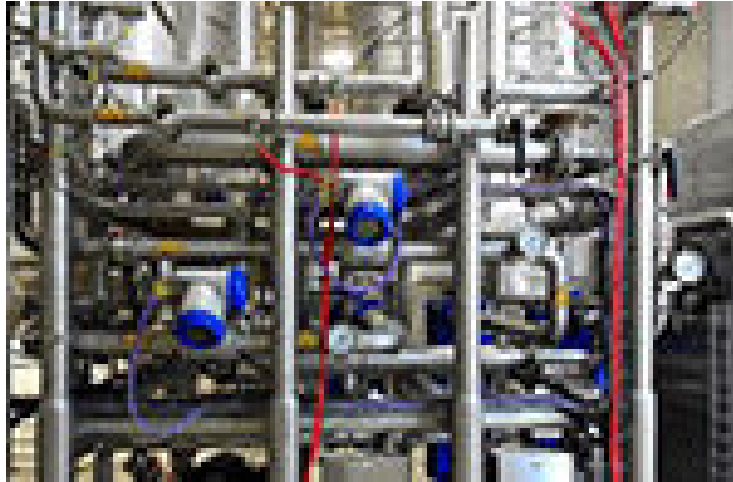
Fig. 6-17 Hot stainless steel piping at a chemical processing plant
