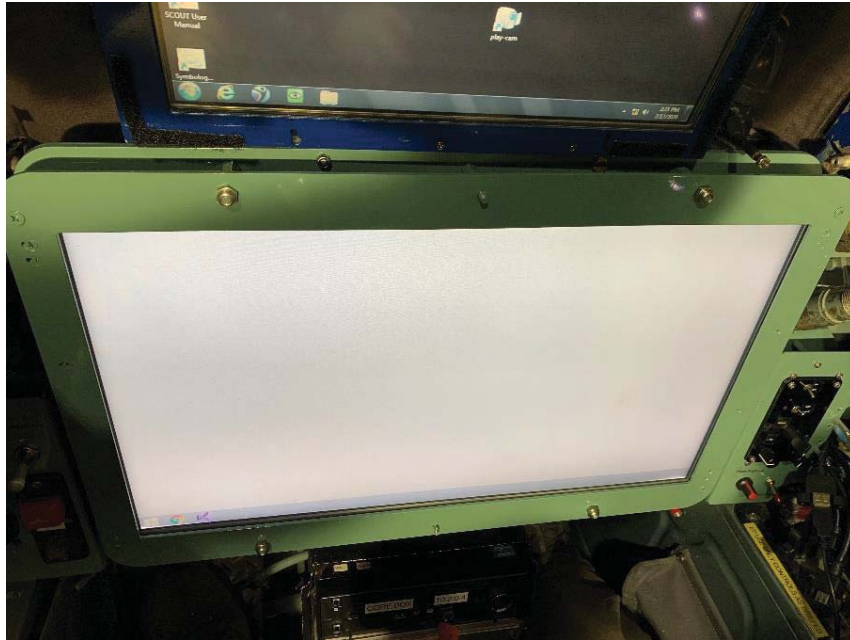
Figure 9. IDK-2121W Touchscreen, Installed
