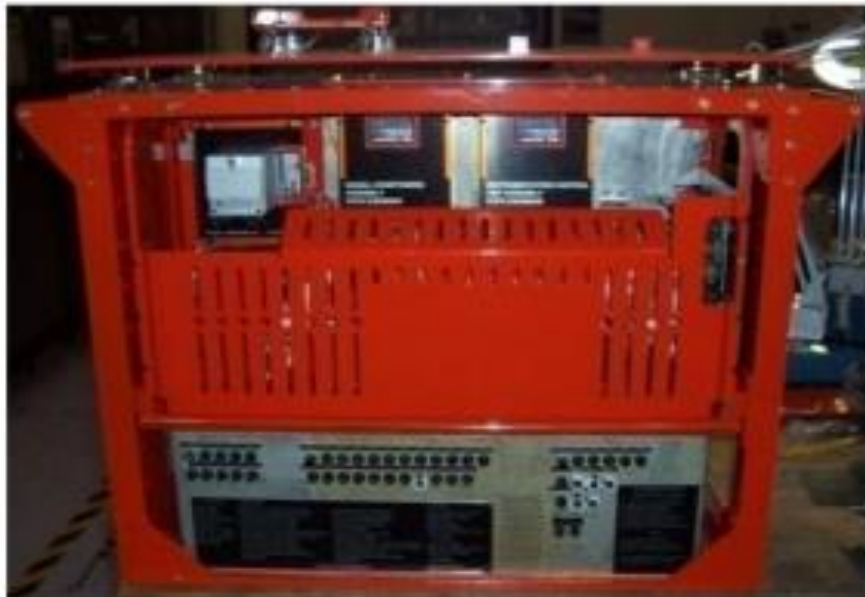
Figure B3. DAS Rack
