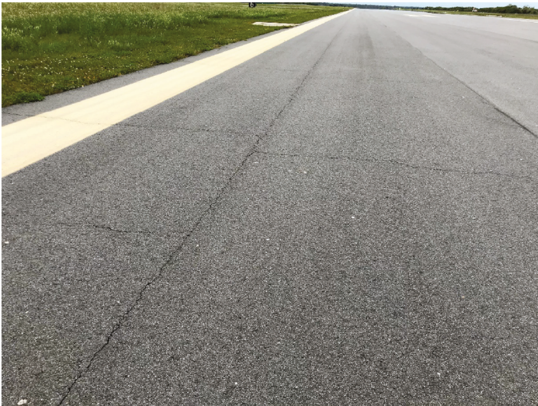
Figure 4. Low severity weathering and cracking on RW 05-23 wing section.
