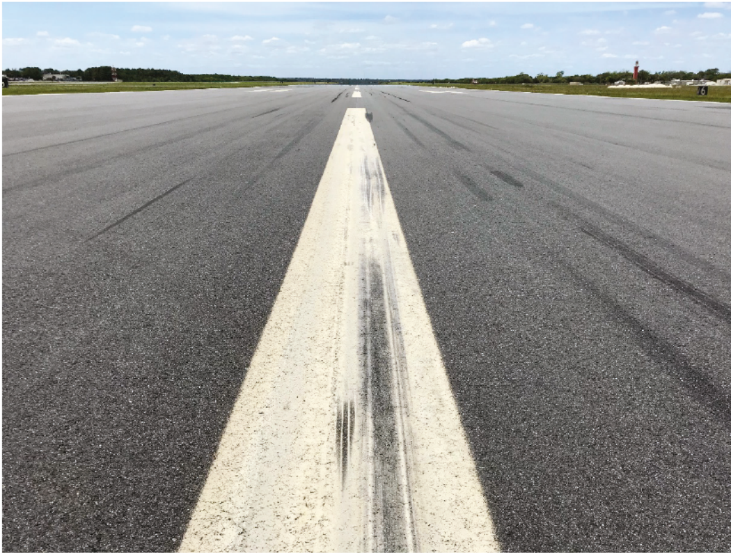
Figure 5. Low severity weathering on RW 05-23 keel section.
