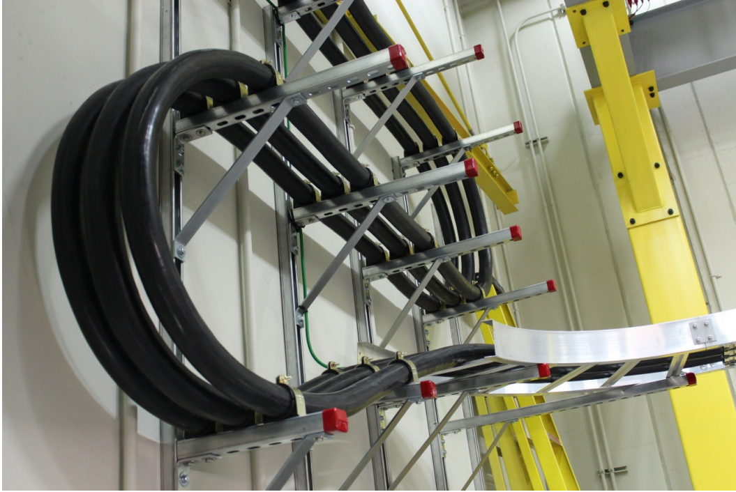
Fig. B-9 Excess variable frequency drive cable lengths were used for Drivelines 1, 2, and 4 to enable reconfiguration
