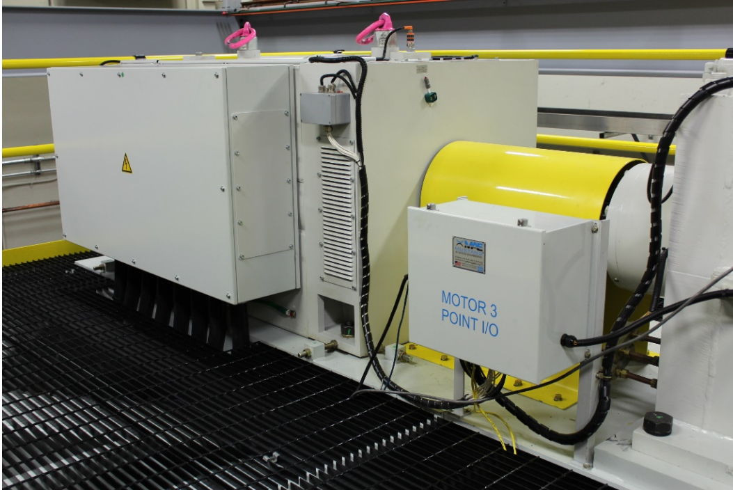
Fig. B-5 Motor 3 absorbs the load from Gearbox 3
