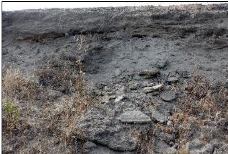
Figure 5. Example of severe embankment weathering on the riverside slope along the Ranch House road segment.
