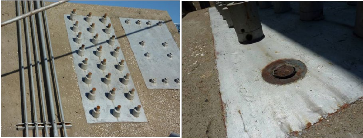
Figure 14. Rod ends at Kaskaskia Lock and Dam (left); broken rod (right).
