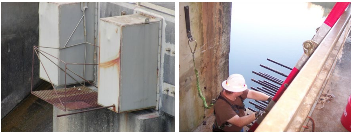
Figure 12. Failed anchor rod penetrating cover, showing one dimple in each cover indicating failed rods that did not penetrate (left); cover removed exposing anchor rods prior to testing (right).
