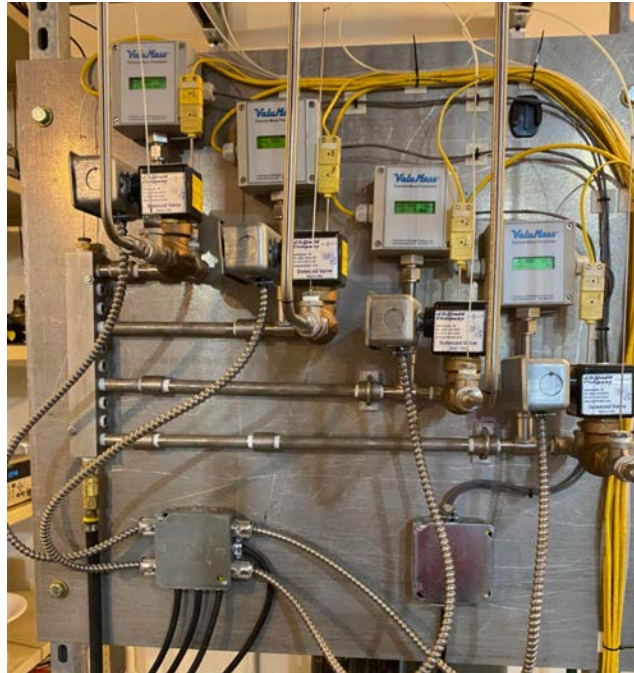
Figure 27. Heat Exchanger Inlet Instrumentation
