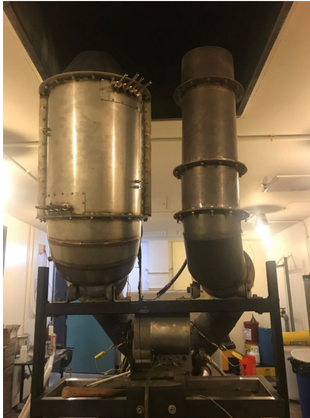
Figure 2. Buck's Fabricated Heat Exchanger Installed. Source: [7].
