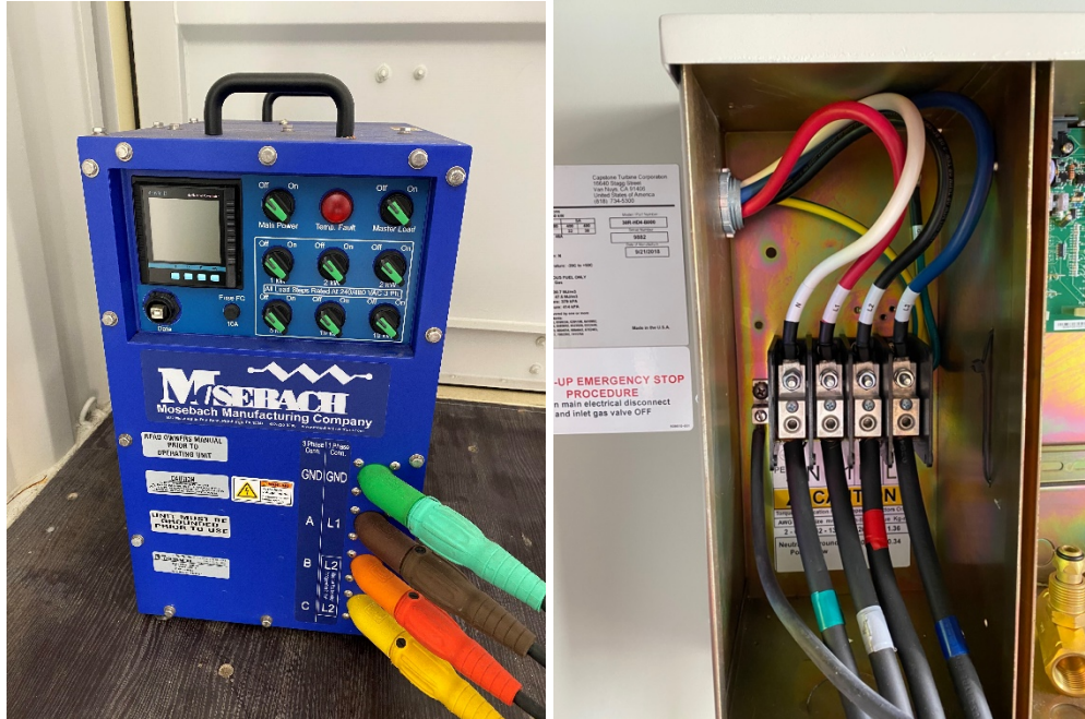
Figure 7. Load bank and end connection to C30.
