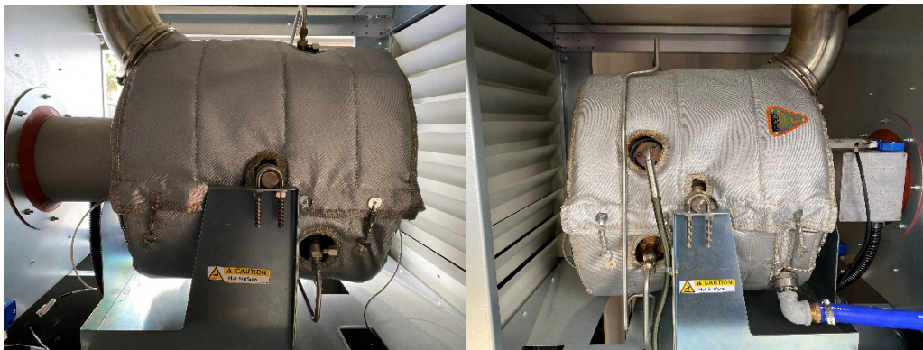
Figure 6. Combustion chamber without pre-mix tubes and capped fittings.
