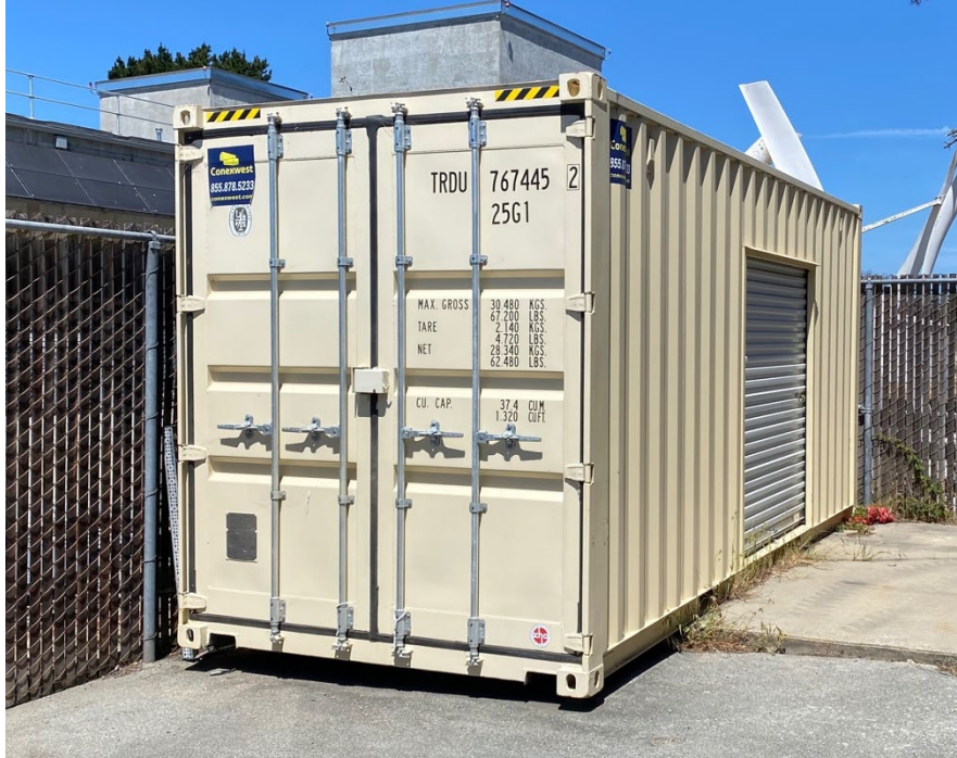
Figure 4. Conex box for C30 and fuel supply system
