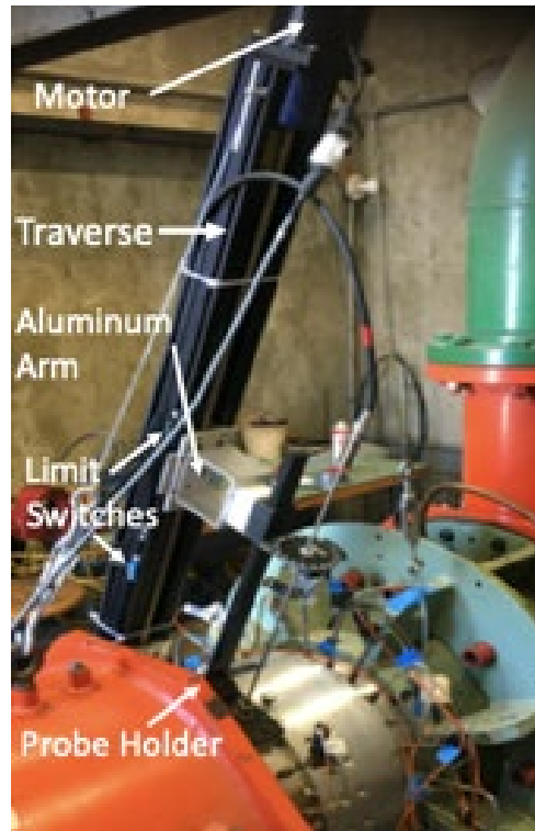
Figure 9. TCR Rig Configuration
