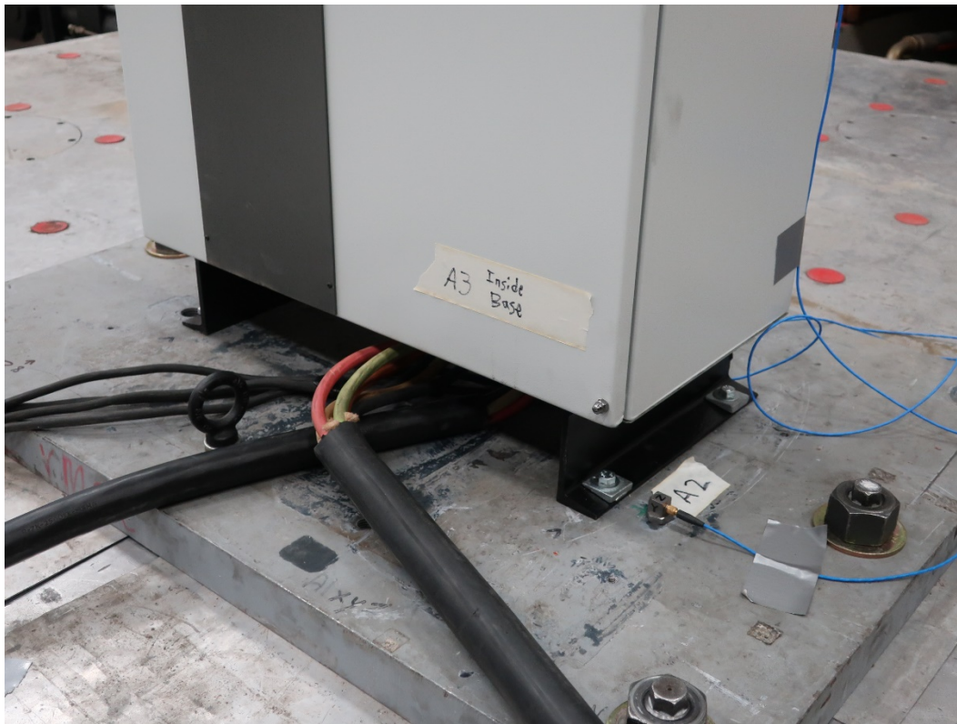
Figure 8. Locations and orientation channels at base of Static Power STS—note the bolt anchoring the channels to the 2 in. (51 mm) plate at the front-right corner .
