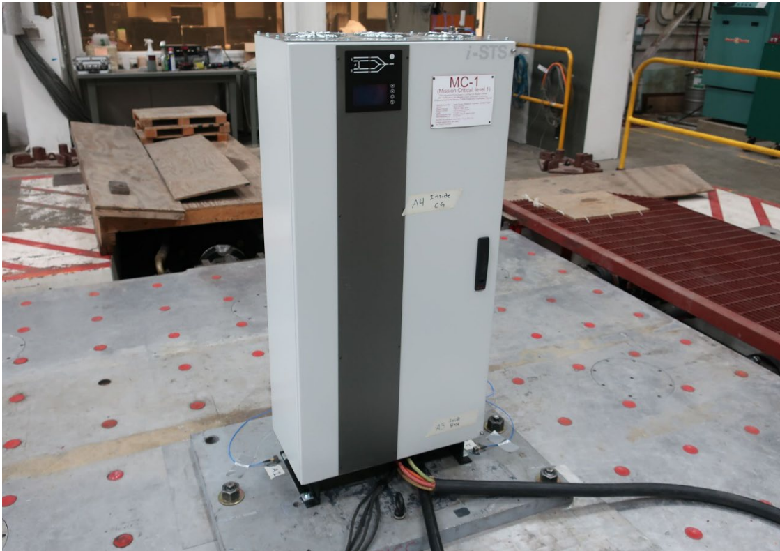
Figure 27. Front view of the STS with the front panel closed and electrical power and load bank connected.
