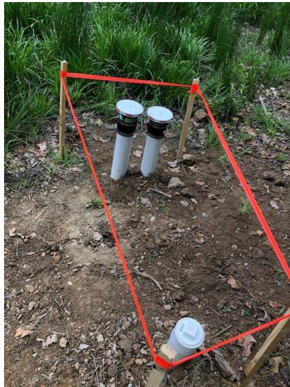
SVP-02 location E-Flux carbon trap installations (top) and soil vapor probe (bottom)
