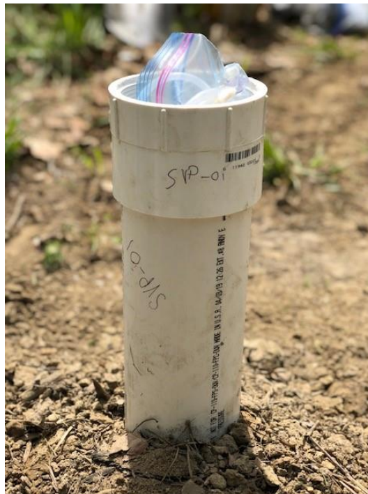
SVP-RC-01 at location RGM-01 (October 2019)
