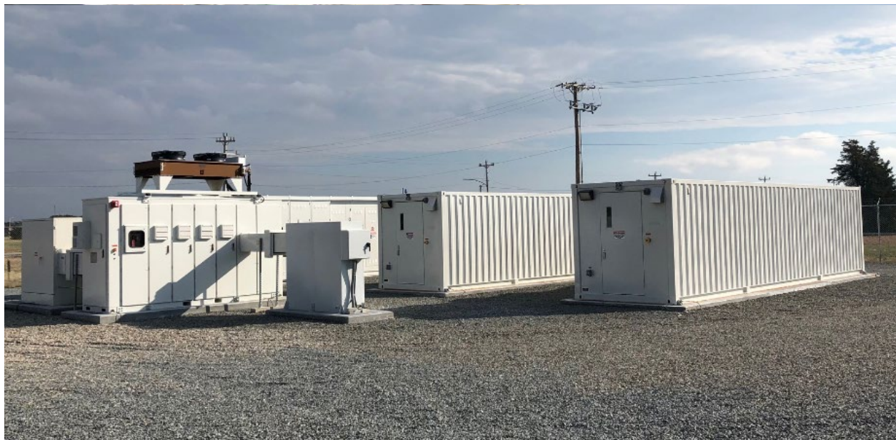
Figure 17. Depiction of Ultrabattery Energy Storage System and Microgrid Switchgear
