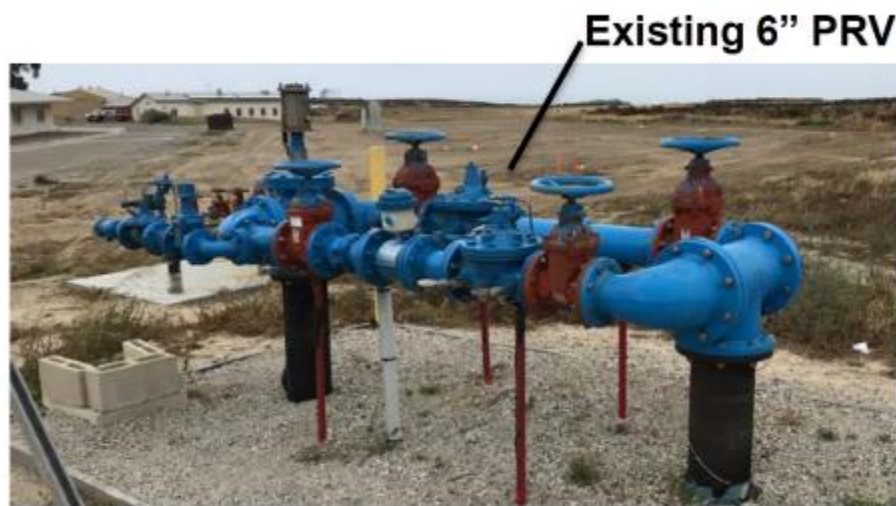
Figure E-2. Image of 6-inch PRV Currently Installed at Nictown
