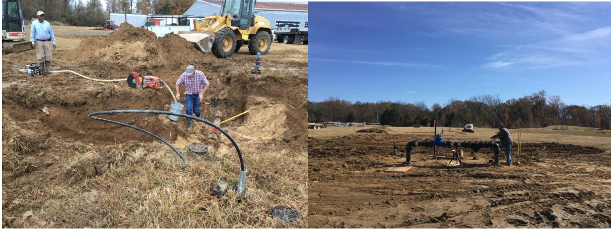
Figure 3-4. Addition of a By-pass During Modification (Left) and After (Right)
