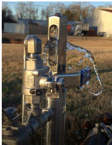
Figure C-9. Ruptured Sight Glass on Cla-Val 98-06
