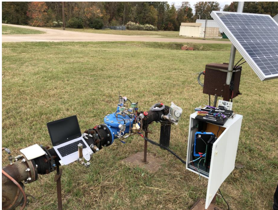
Figure 4-2. Cla-Val 131 Wired Up to VC22-D Controller and Solar
