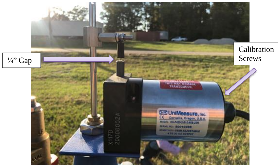
Figure 4-3. Valve Position Transmitter Calibration
