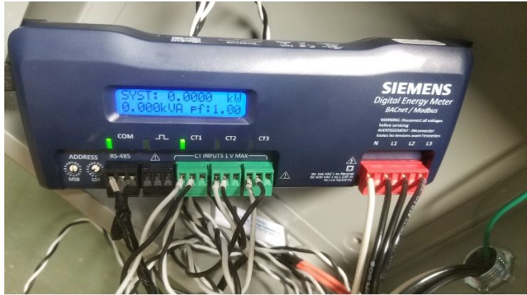
Figure 18. Siemens Power Meter.
