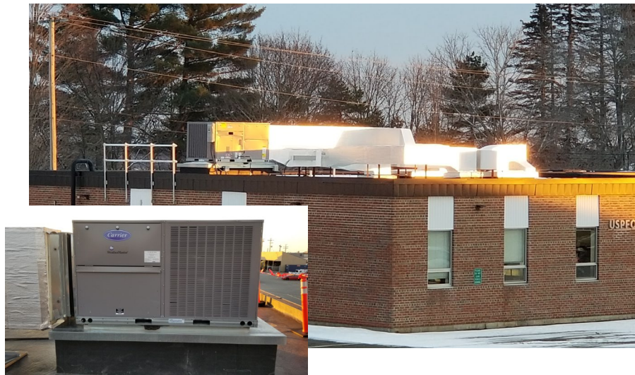
Figure 25. Phase III 7.5TR Cooling and Gas Fired Heating Unit.
