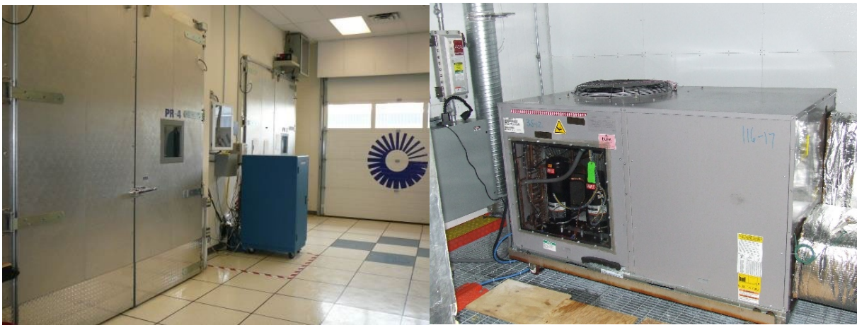
Figure 15. UTRC Psychrometric Facility and Unit#2.
