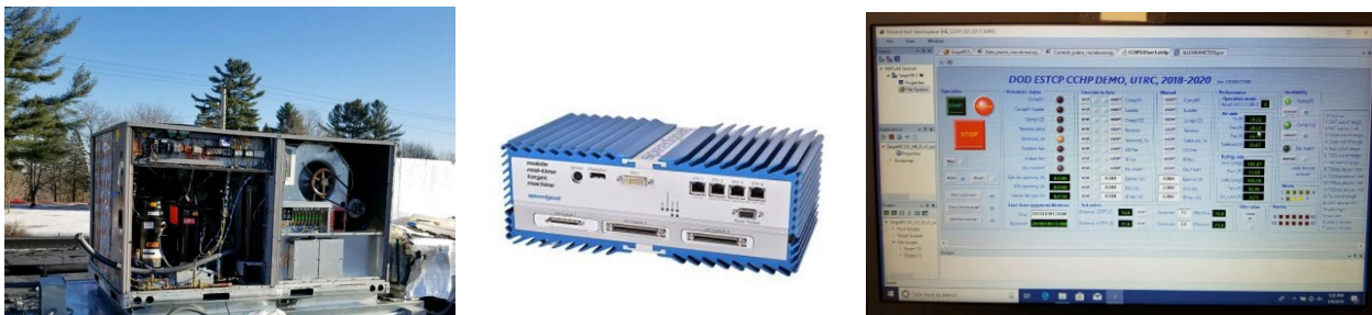
Figure 24. Phase II Advanced CCHP Unit and Controls.
