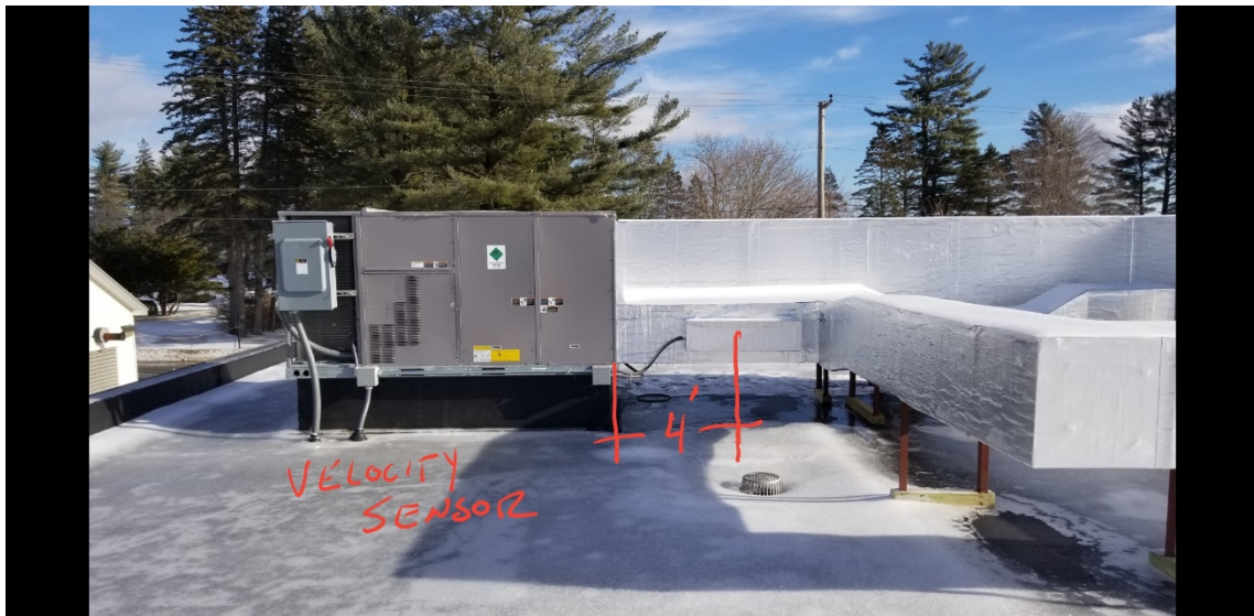
Figure 17. Carrier Heat Pump 50HCQD12 Installed at Camp Keyes.
