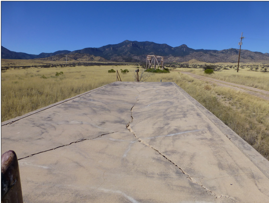
Figure 214. Concrete stairs and cracked platform on top of Facility 16303 (ID #29) (ERDC-CERL 2016).
