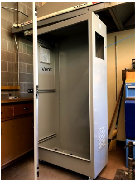
(a) Control system enclosure
