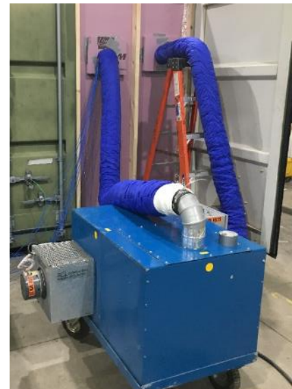
Figure C-2. 250K BTU GFE heater used for Trials 1-3
