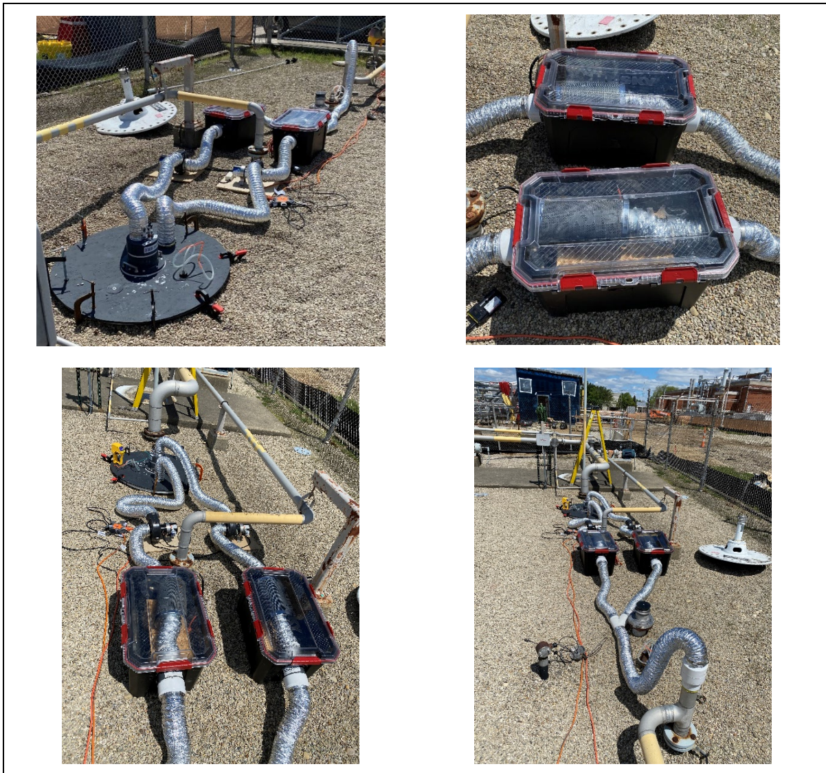
Figure 55. Dual activated carbon filter/tote system for in-line gas neutralization
