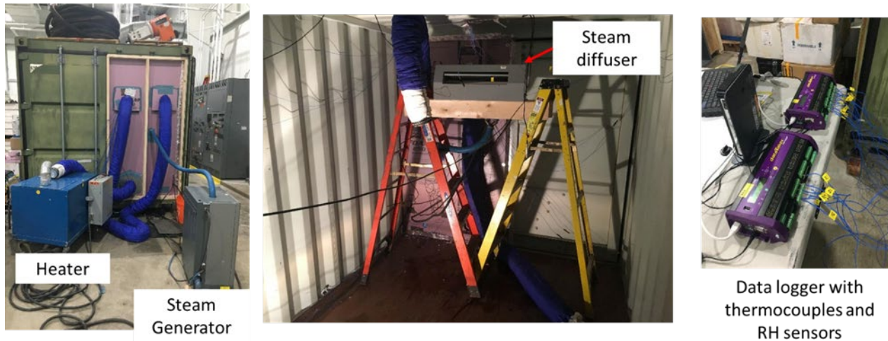
Figure 25. Test system used for HAD Mock-up Trials 1-3: 250K BTU heater and Carel steam generator shown in left image; steam diffuser placed inside the shipping container and connected to an exterior steam generator (middle image); and thermocouples and RH sensors connected to data loggers (right image).
