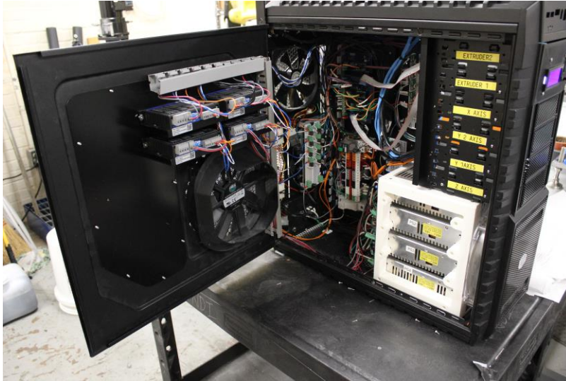
Figure 2 Electrical controller enclosure
