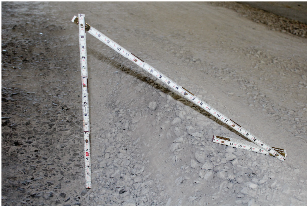
Figure 24. Depression at transition from Item 2 (NX750) to Item 3 (unstabilized).
