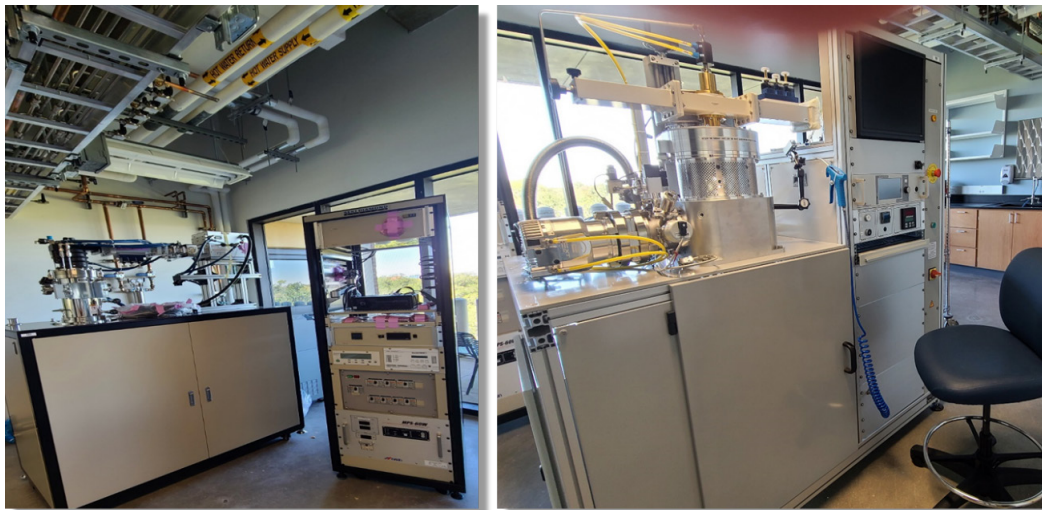
Fig. 5 Diamond growth MPCVD systems, SEKI SDS6350 (left) and Plassys SDR-150 (right), being installed at the facility
