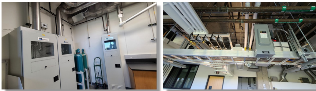
Fig. 4 Infrastructure installation underway; gas safety cabinets for H 2 , methane, and ammonia storage (left), and a segment of the infrastructure rack at the ceiling, carrying electrical, gas, coolant, and compressed air lines
