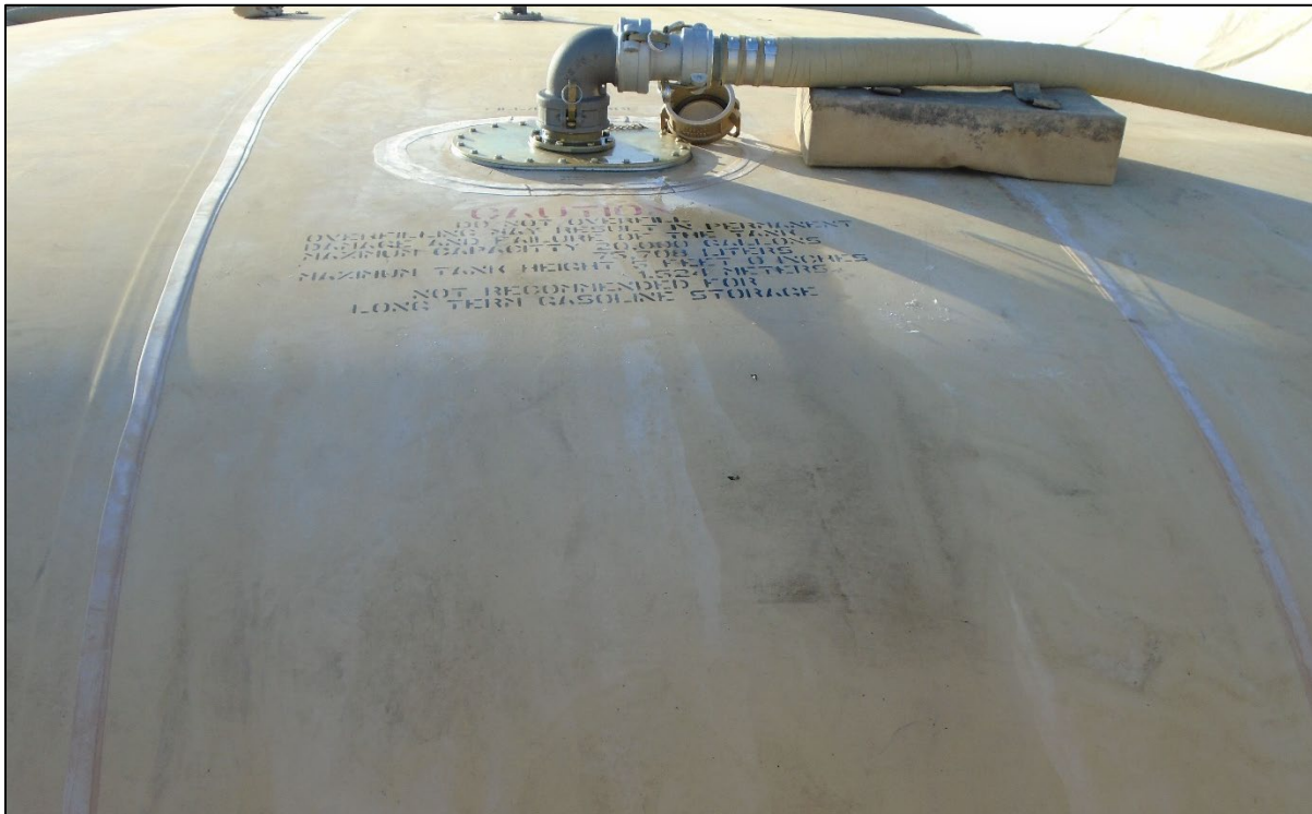
Figure E-4. AEF #5 CFT Fuel Leak from Stripped Bolt at Port Flange
