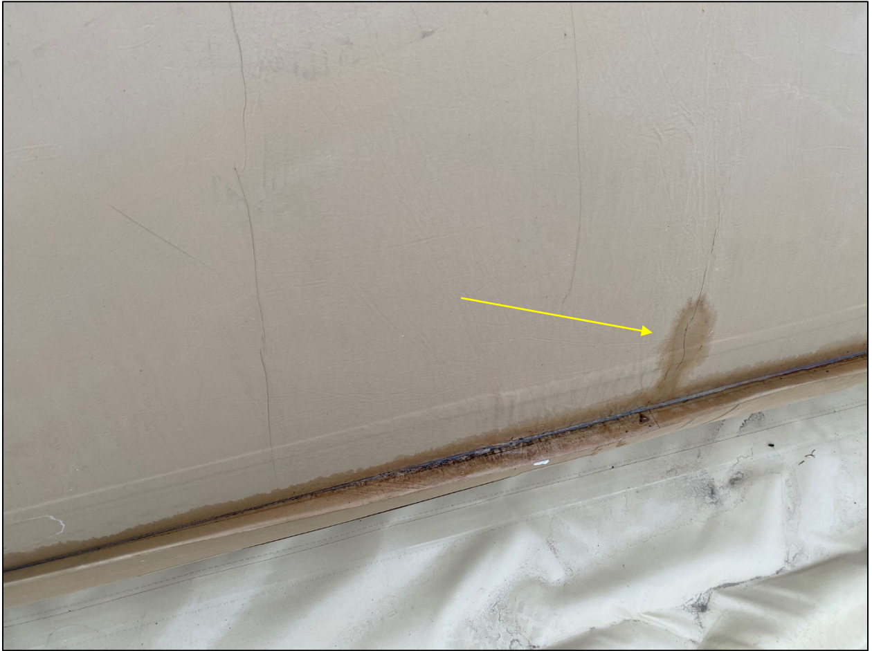
Figure A-9. BLSS #1 (NAFT #1) Fuel Leak from Surface Crack and Pooled Along Edge
