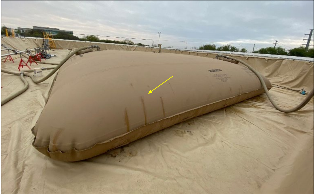
Figure A-7. BLSS #1 (NAFT #1) CFT Fuel Leaks and Drips
