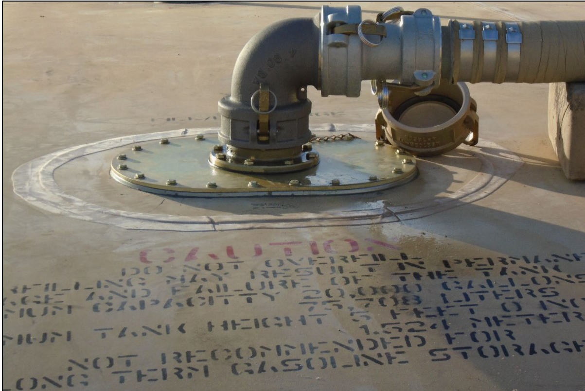
Figure E-3. AEF #5 CFT Fuel Leak from Stripped Bolt at Port Flange
