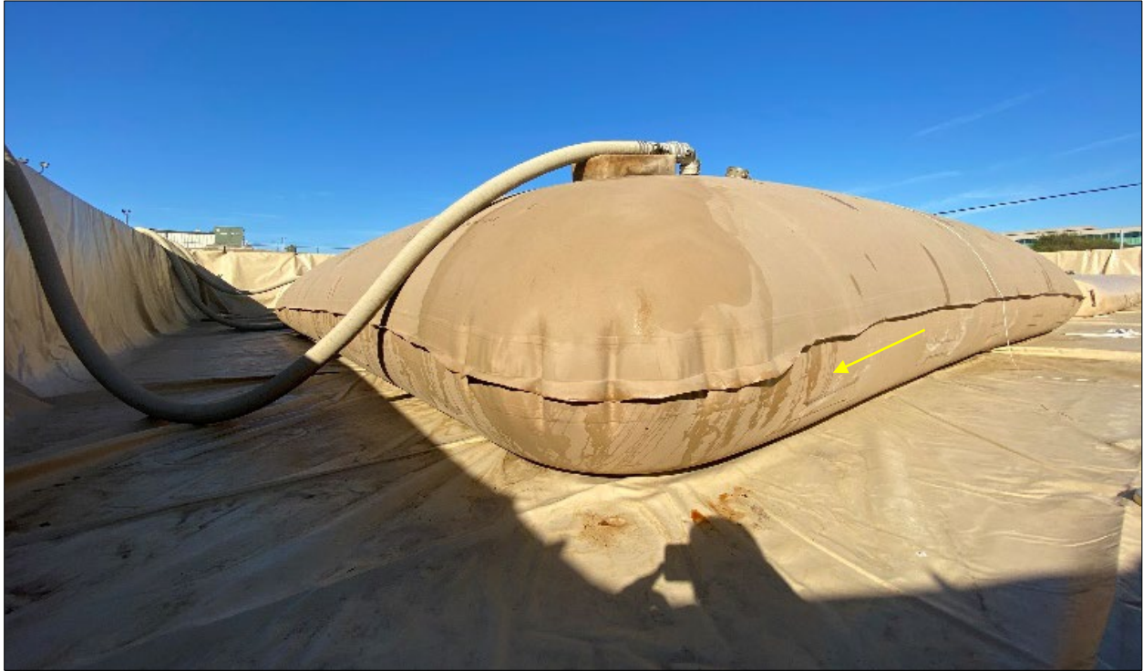
Figure A-5. BLSS #1 (NAFT #1) CFT with Fuel Leaks Below Seam
