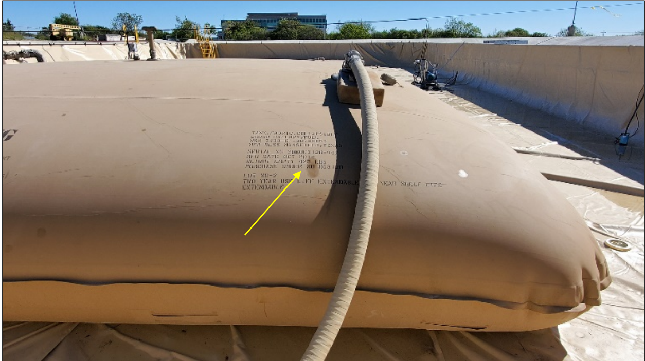
Figure A-3. BLSS #1 (NAFT #1) CFT with Fuel Leak Through Fabric
