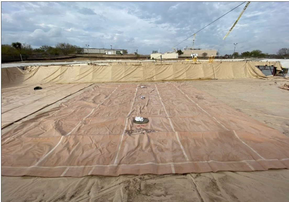
Figure B-4. JGB #2 NITRILE CFT Unfolded and Deployed (Looking North)
