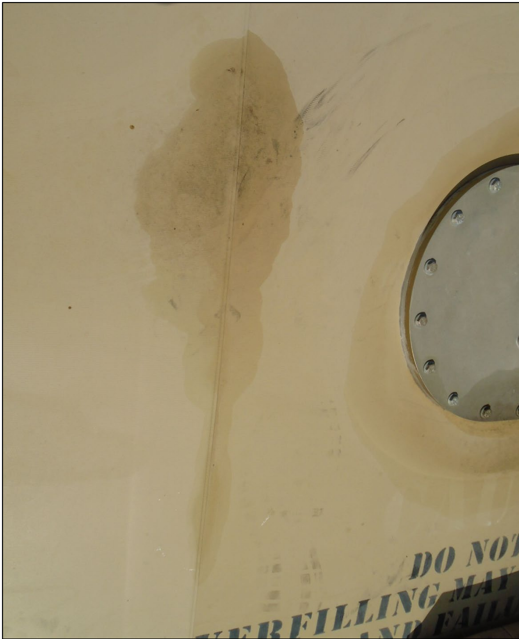
Figure D-11. MILPAWS #4 CFT at End of Test Program Showing Seam Leak
