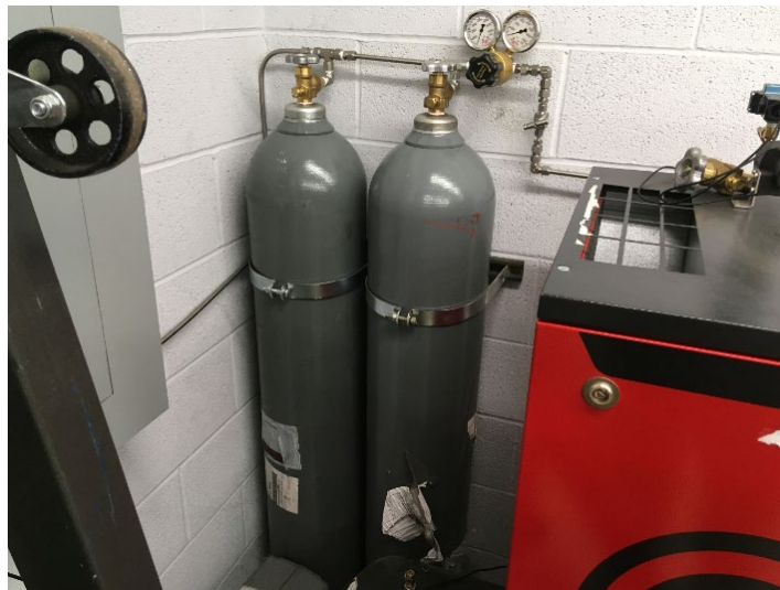
Figure 21. Compressed Dry Air Storage Tanks. Source: [1].
