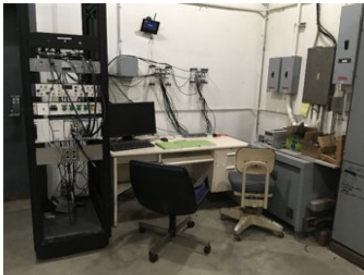
Figure 25. Light Gas Gun Control Room. Source: [1].
