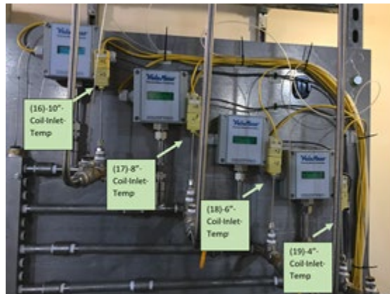
Figure 12. Coil Inlet Thermocouples
