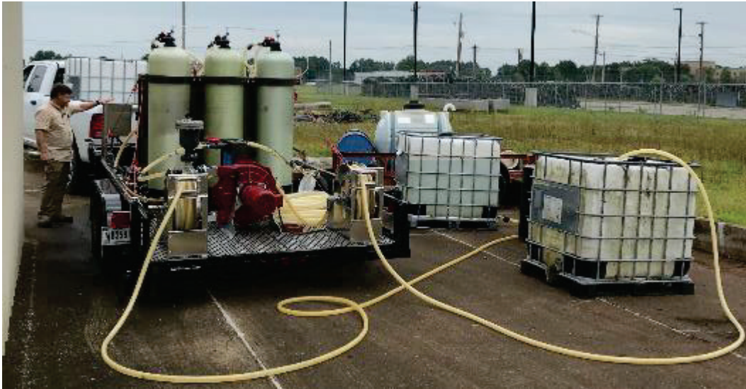
Figure 3. PFAS Effluent Treatment System (PETS).
