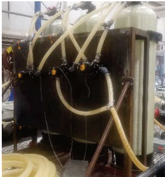
Figure 15. Media tank support frame.
