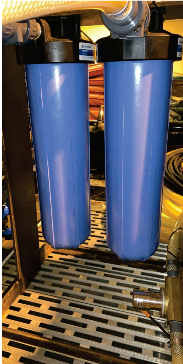
Figure 16. Sediment filters and support frame.
