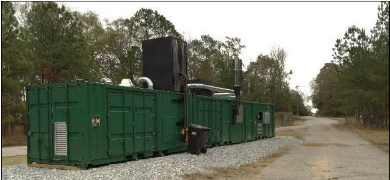
Figure 42. Photograph of the BWEC system during demonstration at Ft. Benning
