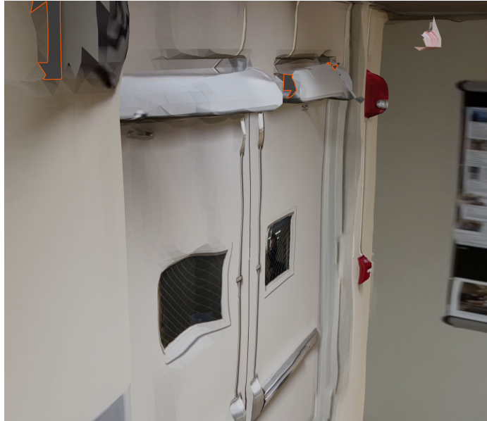
Figure 12: More blemishes that could be corrected. Note the holes and the warping in the door.
