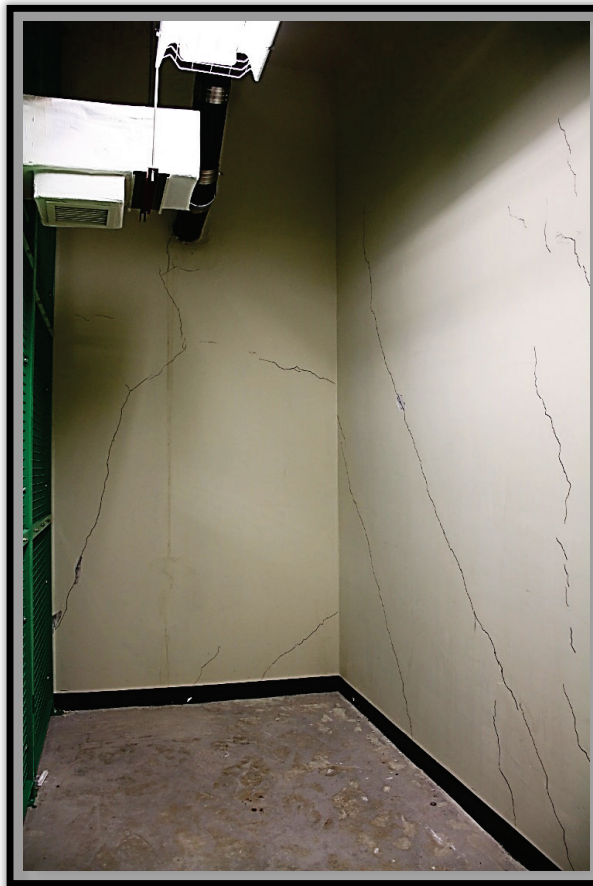
Figure B19. Mapped diagonal cracks in basement storage area of Tower 2.
