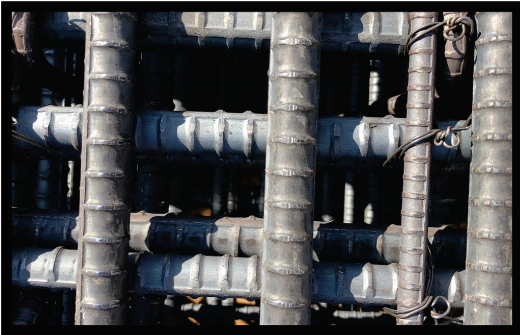
Figure 38. Rebar congestion in slab-beam intersection in Parking Garage 4.
