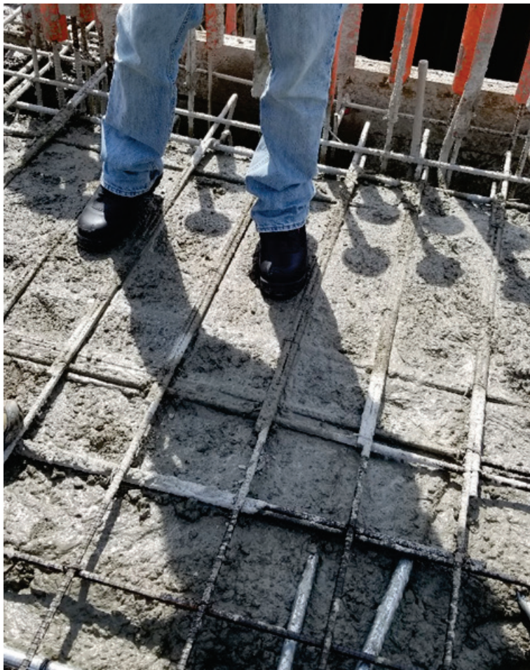
Figure 35. Concrete placement terminated within a slab. The person standing on the concrete indicates that this concrete has hardened.
