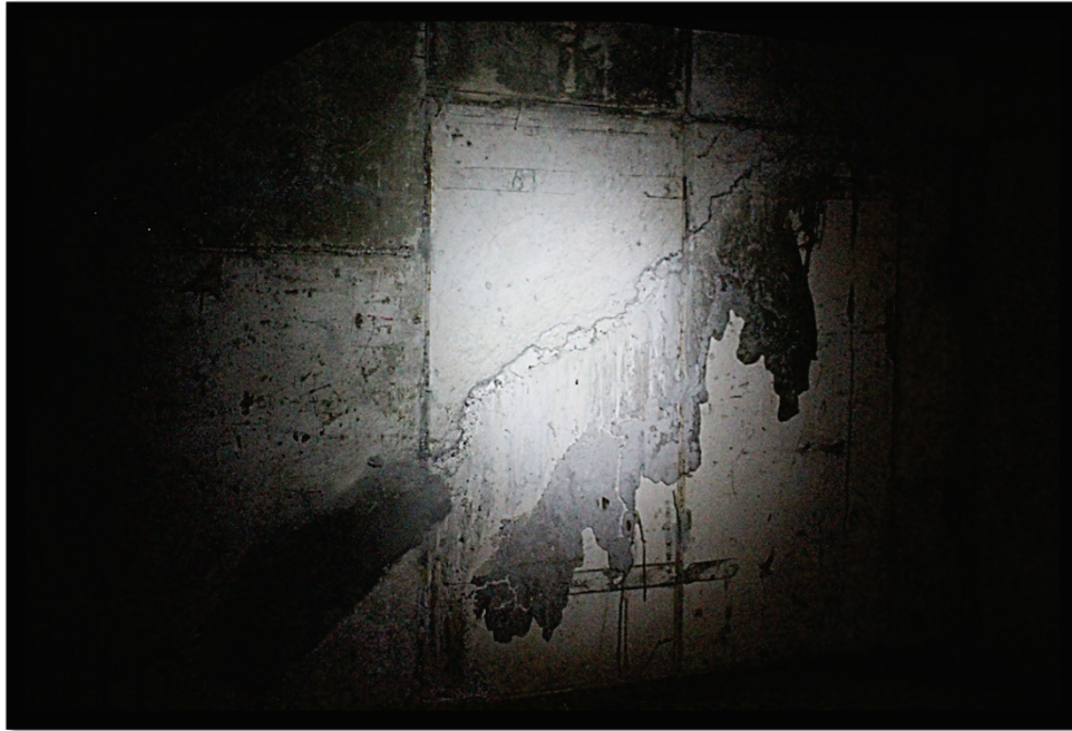
Figure 58. Diagonal cold joint under staircase in Parking Garage 4.
