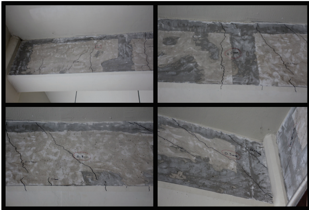
Figure B60. Mapped cracks in bare concrete of beam along column line 4 in Parking Garage 1.
