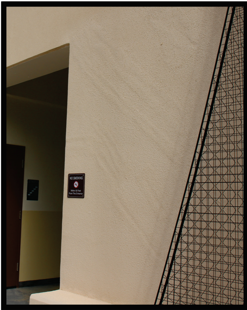
Figure 53. Repaired diagonal concrete cracks visible beneath exterior coating on Parking Garage 3.
