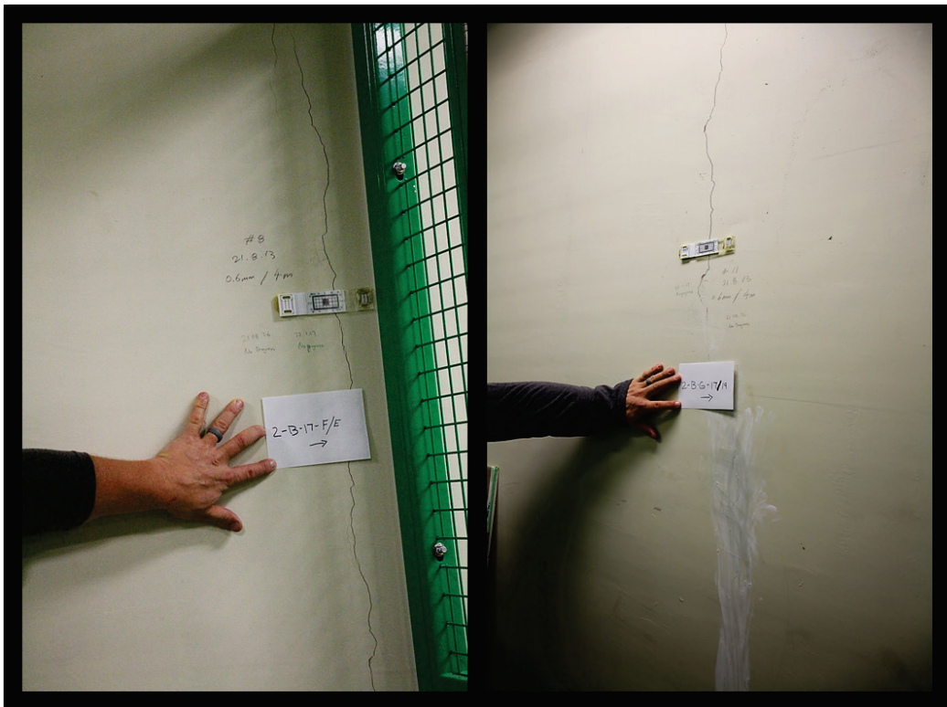
Figure B15. Wall cracks with gauges in Tower 2 basement.
