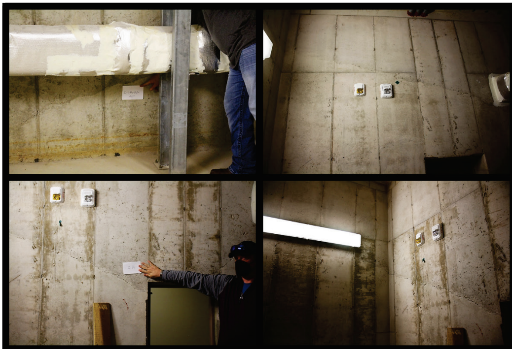
Figure B23. Cold joints in shafts behind elevators in Tower 2.
