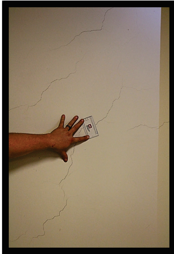
Figure B3. Cracking in mapped wall of elevator mechanical room in Tower 1.
