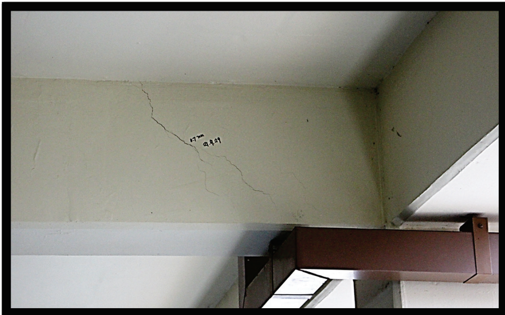
Figure 50. Most severe diagonal crack noted in Parking Garage 2 (0.7 mm).
