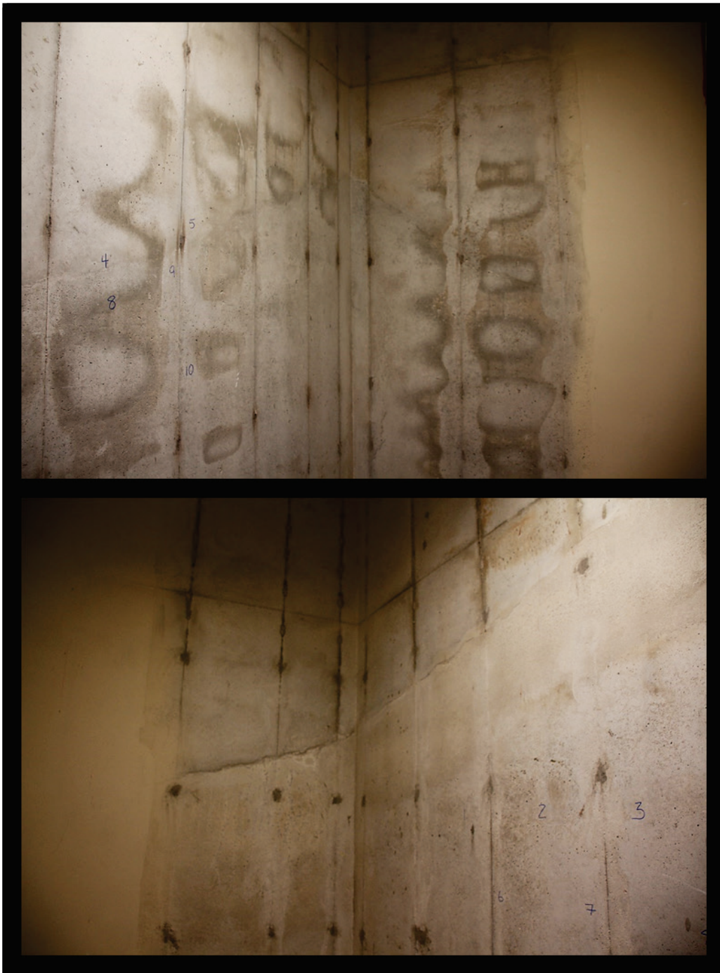
Figure B33. Cold joints in walls of shaft behind the elevators in Tower 3.
