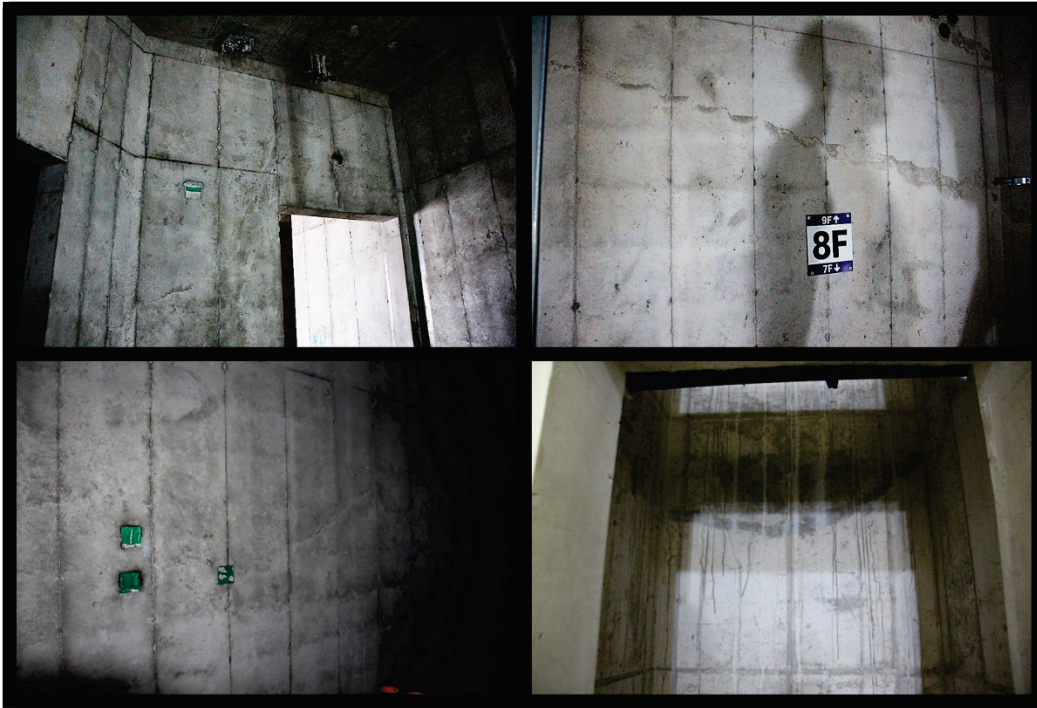
Figure B42. Cold joints in walls of Tower 4.
