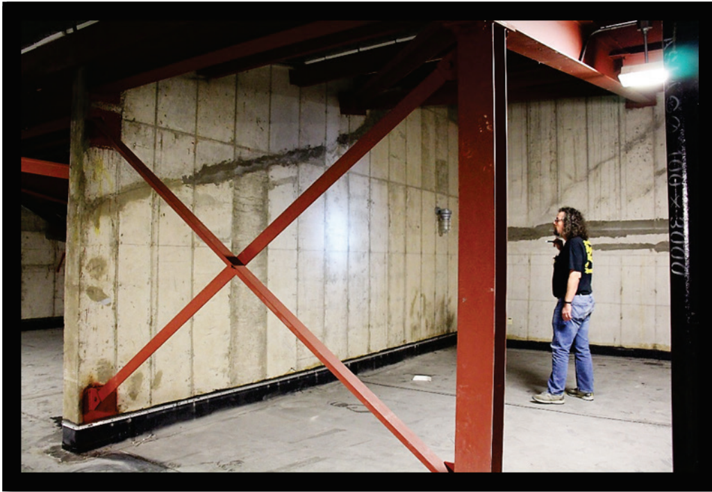
Figure B26. Diagonal cold joint in wall of attic in Tower 2.
