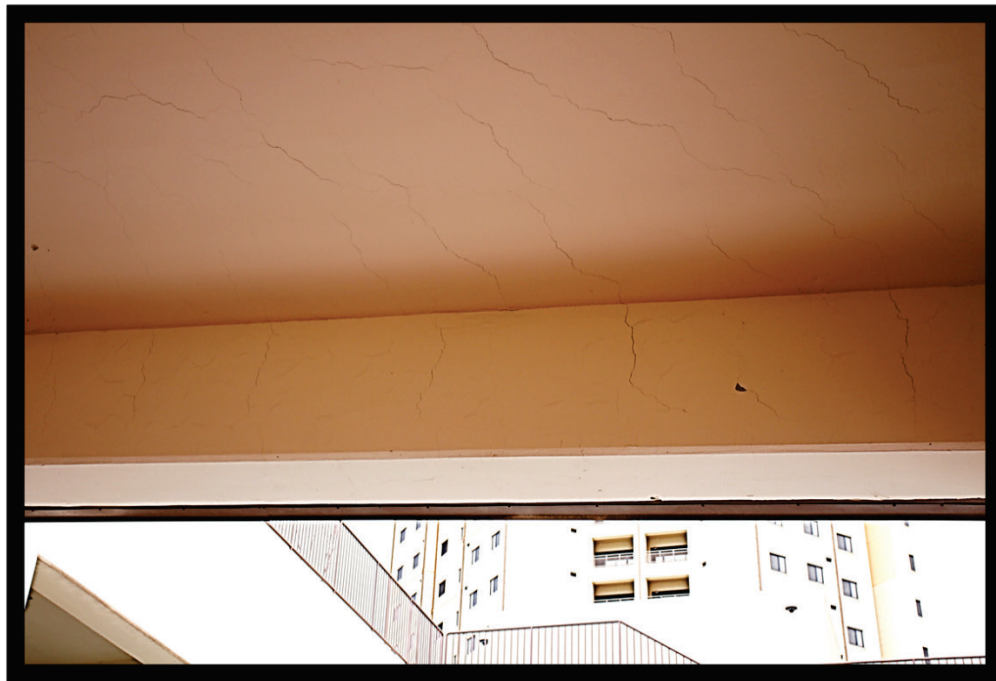
Figure 51. Multidirectional cracking extending from beams into ceiling slab of roof over ramp to floor 2.
