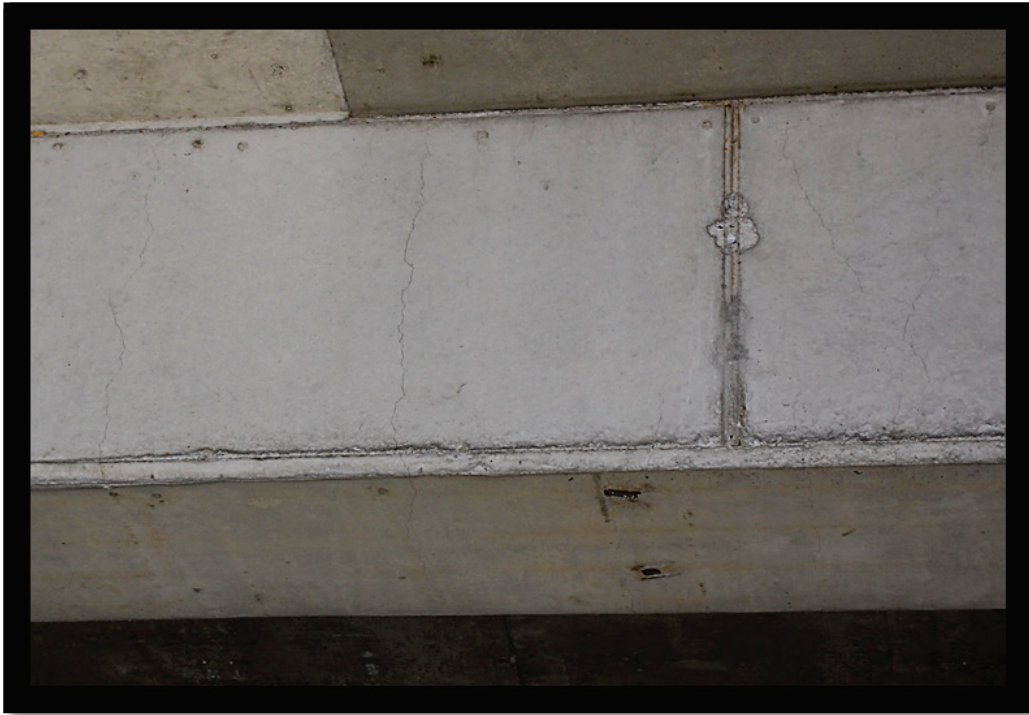
Figure B70. Vertical cracks in beam in Parking Garage 4.
