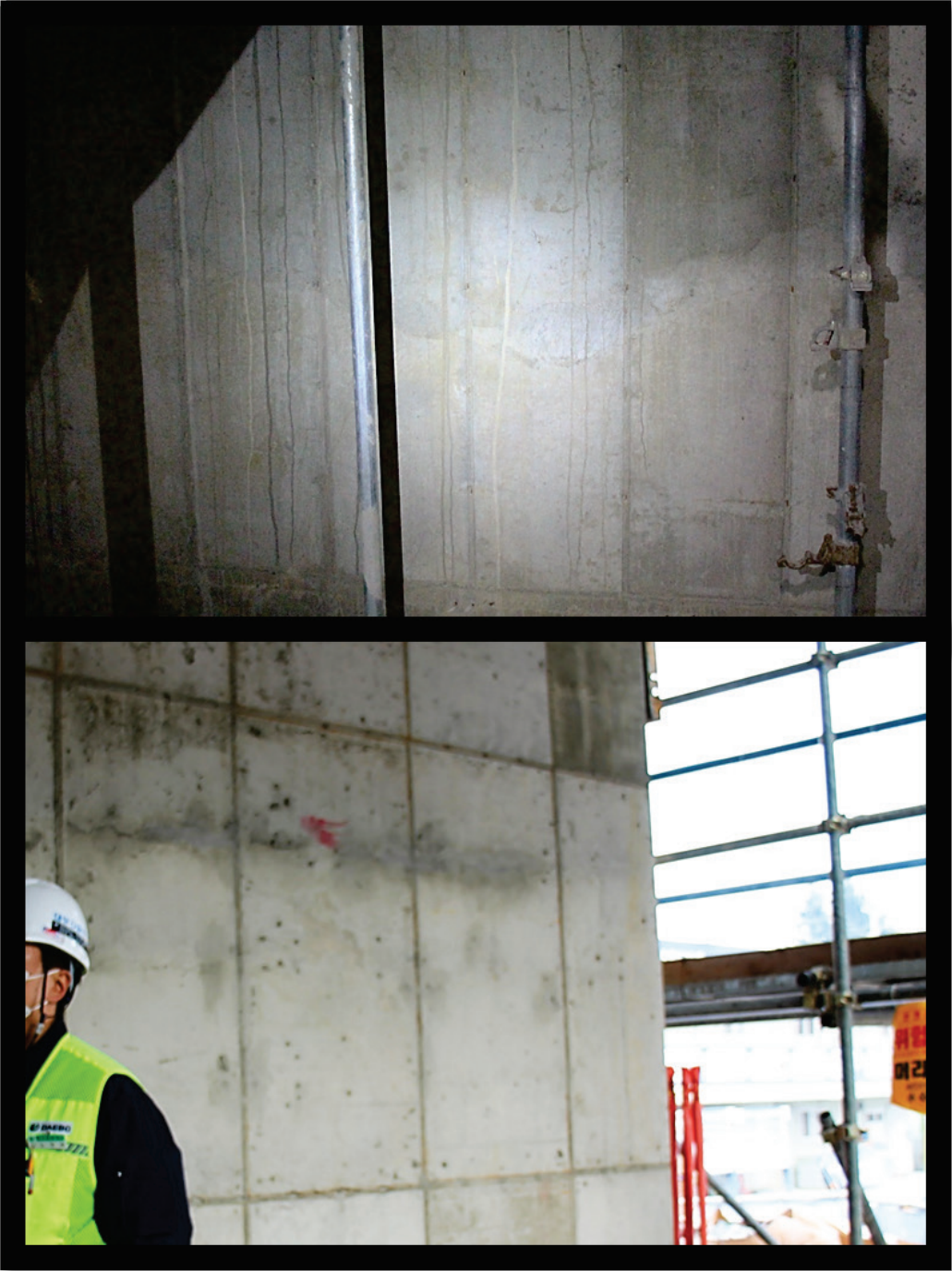
Figure B68. Cold joints in walls in Parking Garage 4.
