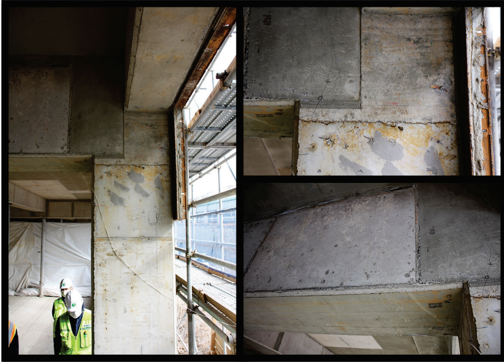
Figure B72. Cracks in exterior column and connected girder in Parking Garage 4.
