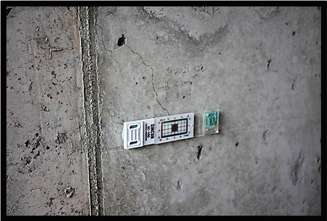
Figure 55. Crack monitoring in Parking Garage 4.
