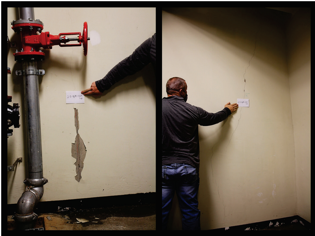
Figure B21. Cracks in basement mechanical room of Tower 2.
