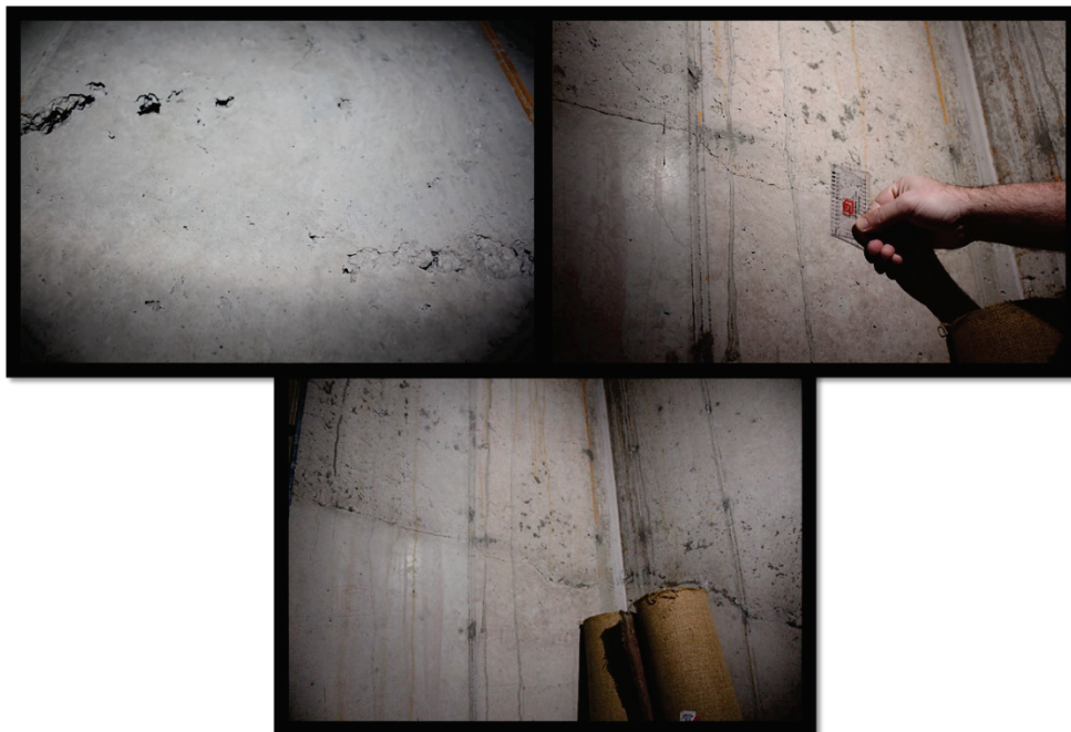
Figure B2. Honeycombing and cold joint in cored shaft of Tower 1.
