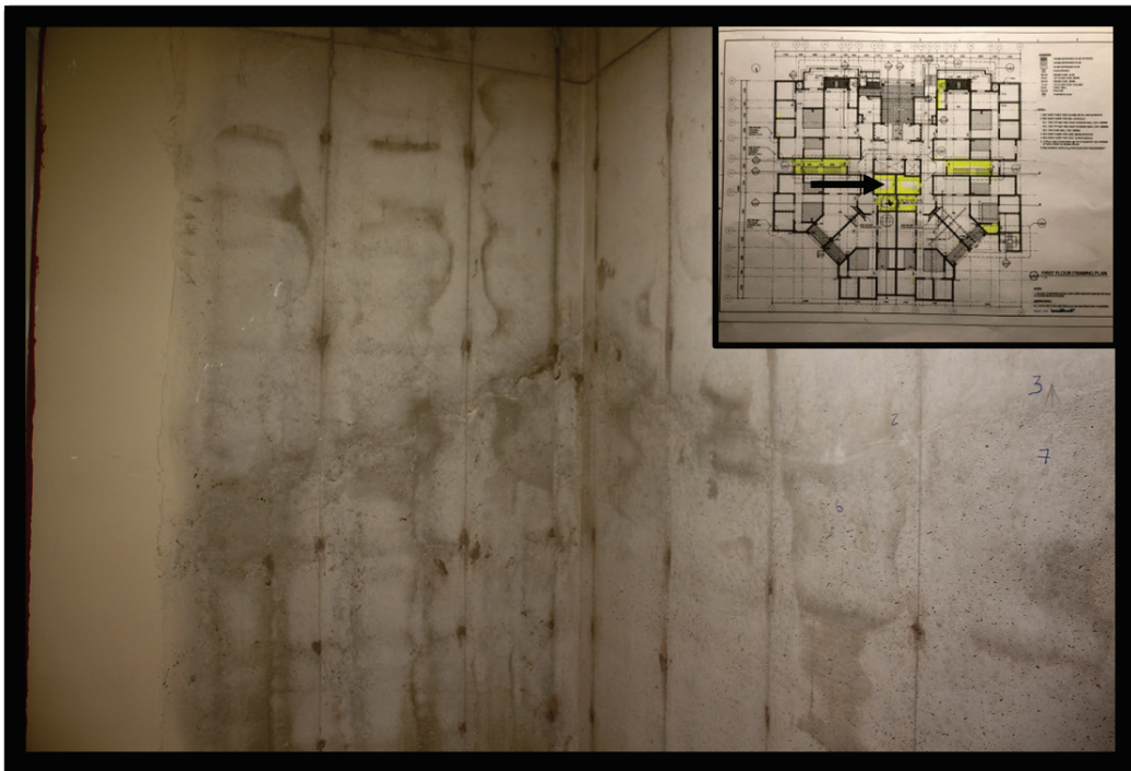
Figure 23. Typical observed cold joints within Tower 3 elevator shaft area (floorplan insert).
