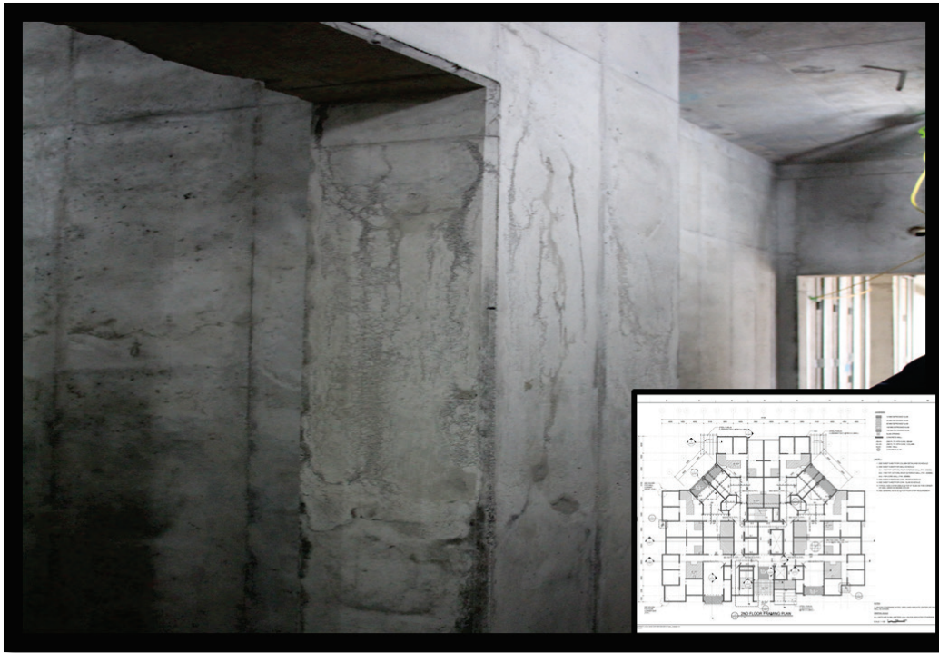
Figure 34. Nonuniformity in Tower 4 concrete wall (floorplan insert).
