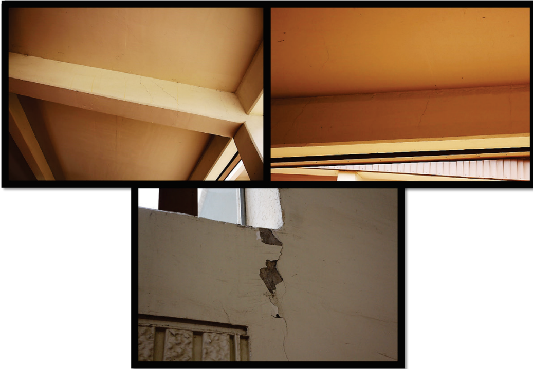
Figure B54. Cracks in ceiling, beams, and wall of entrance to basement of Parking Garage 1.
