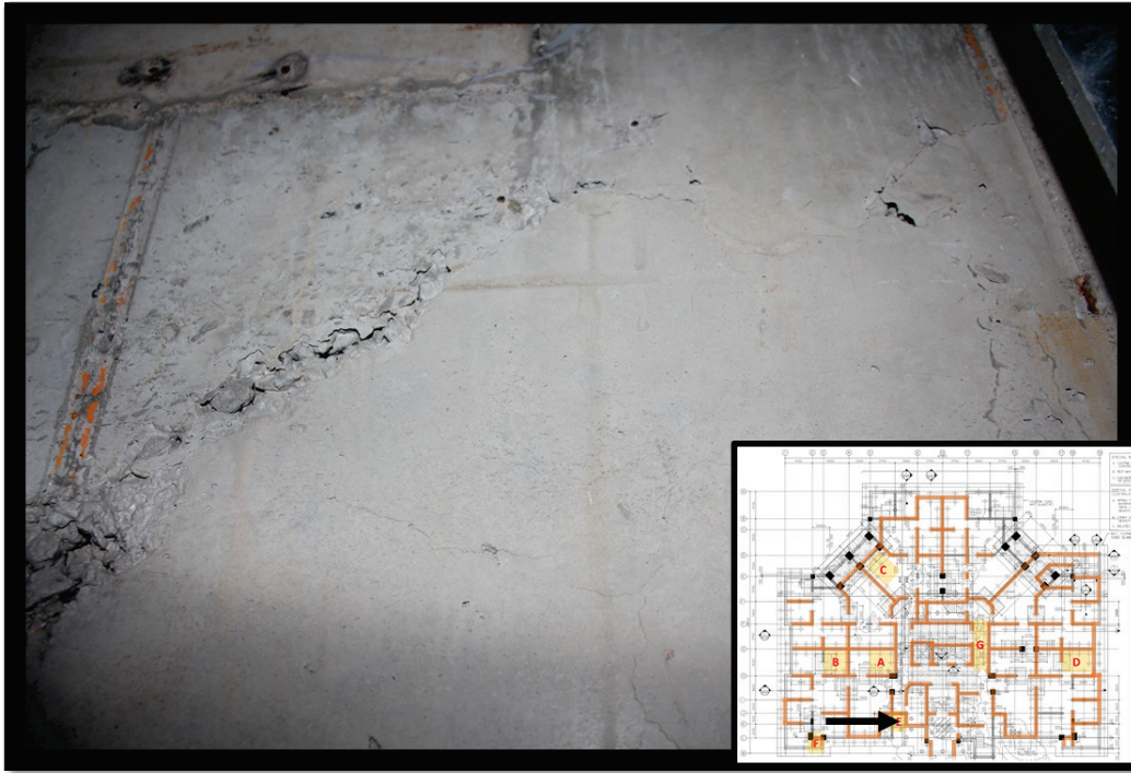
Figure 7. Cold joints within the Tower 1 basement shaft area (Section E of the floorplan insert). These cold joints were observed on bare concrete and were typical in the mechanical and electrical shaft areas in the upper floors.
