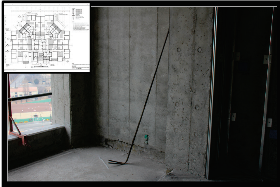
Figure 32. Poor consolidation along bottom wall of Tower 4 balcony and adjacent columns (floorplan insert).
