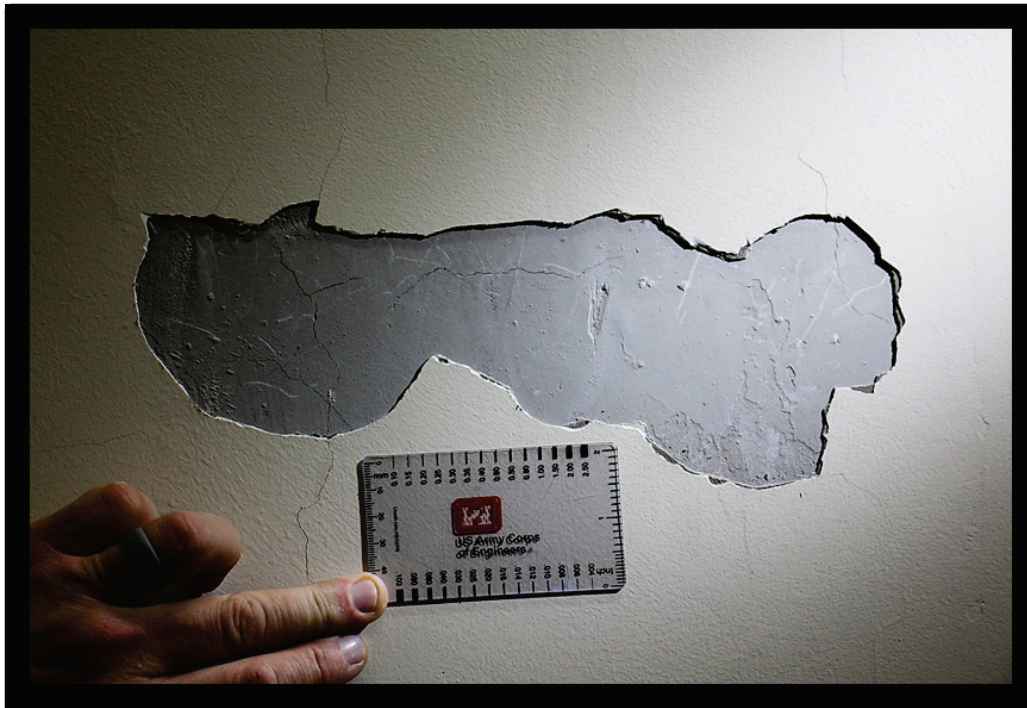
Figure B4. Cracking in concrete and cementitious coating in wall of Tower 1.
