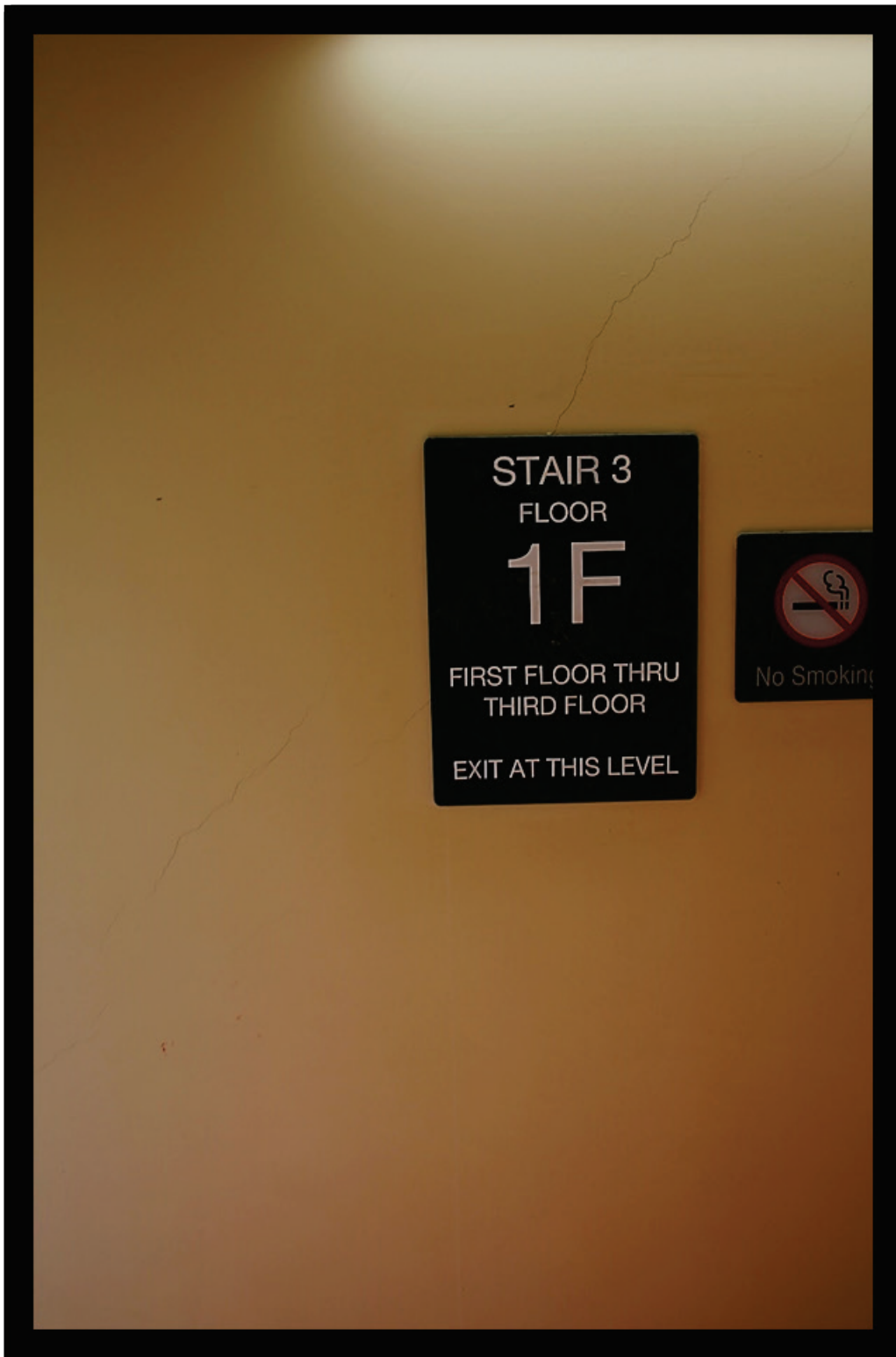
Figure B66. Diagonal crack in wall of stairwell in Parking Garage 3.
