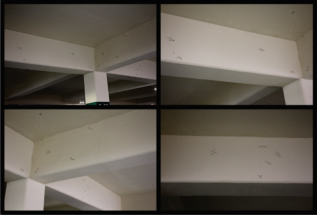
Figure B64. Diagonal cracks in girders and beams in Parking Garage 2.
