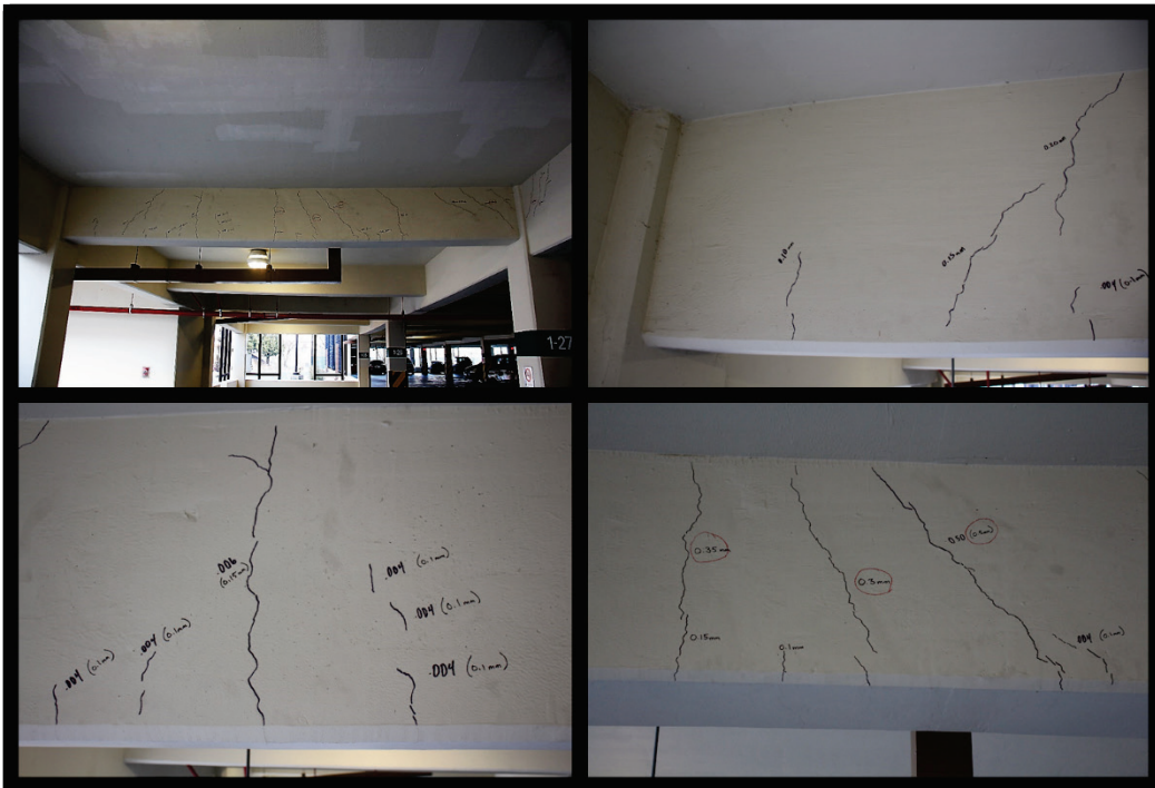
Figure B55. Mapped cracks in beam along column line 4 in Parking Garage 1.
