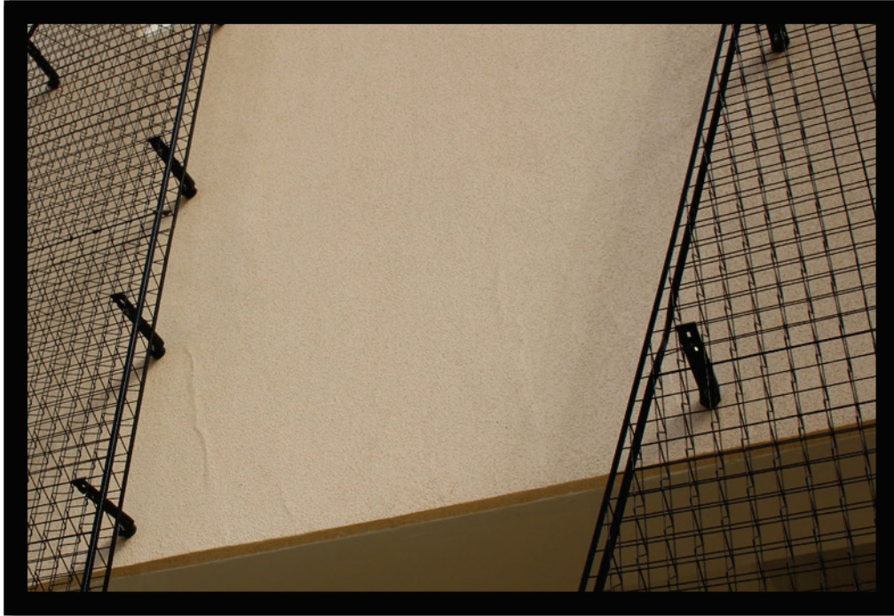
Figure B65. Vertical cracks manifest in surface architectural coating on exterior of Parking Garage 3.
