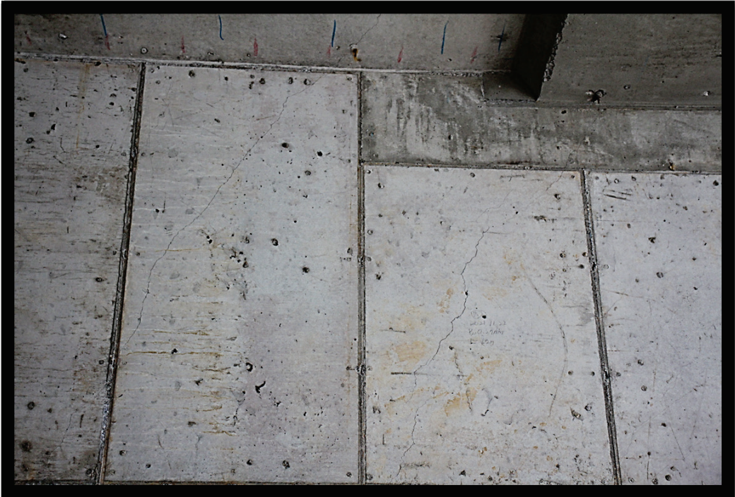
Figure 54. Vertical cracking in stairwell wall of Parking Garage 4.
