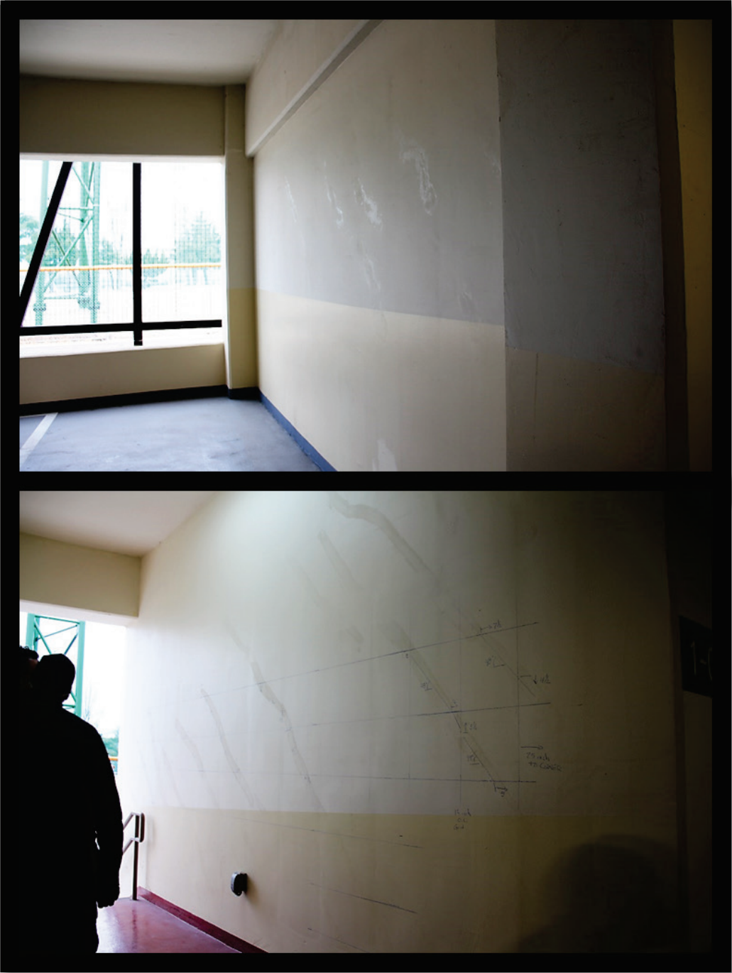
Figure B53. Diagonal cracks in walls in Parking Garage 1.
