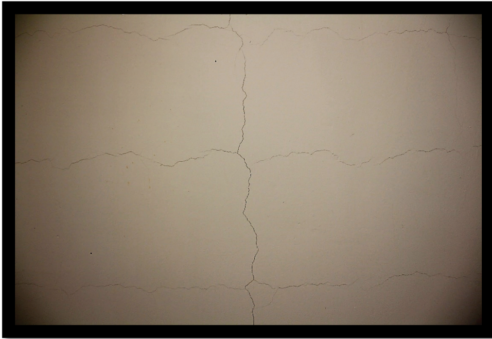
Figure B20. Vertical and horizontal cracks in stairwell wall of Tower 2.
