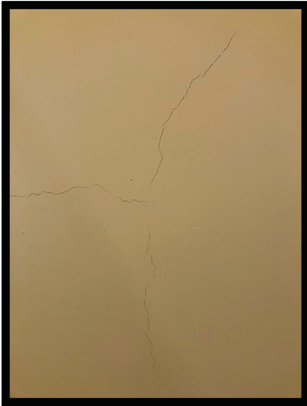
Figure B31. Vertical and horizontal cracks in basement wall of Tower 3.
