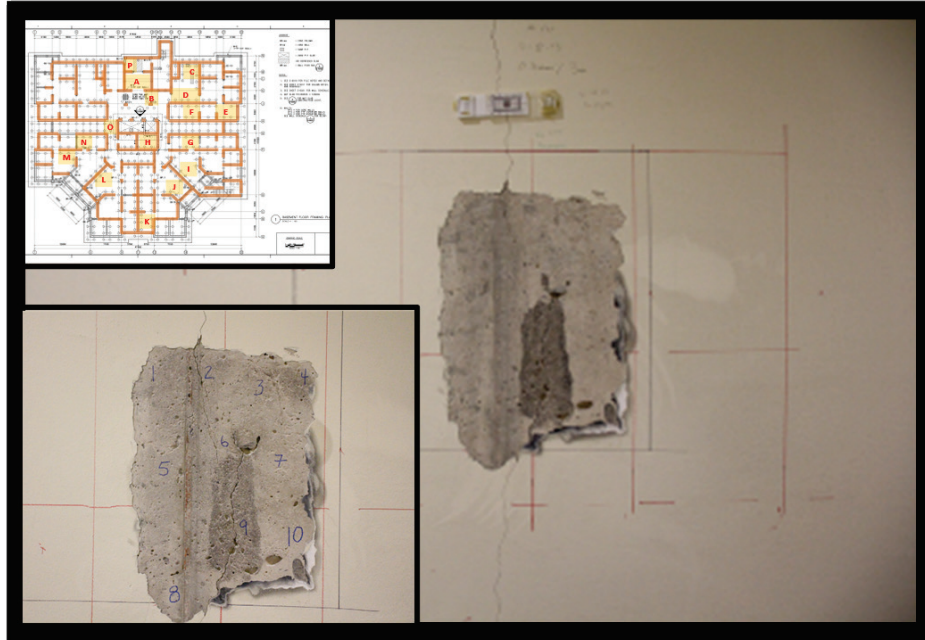
Figure D5. Prepared area for concrete coring in Tower 2. One core was taken over the crack, and two cores were taken to the sides of the crack to be representative concrete samples. Red lines indicate locations of internal reinforcement. Insert shows Schmidt hammer locations.
