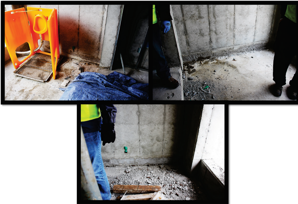
Figure B43. Poor consolidation at balconies of Tower 4.
