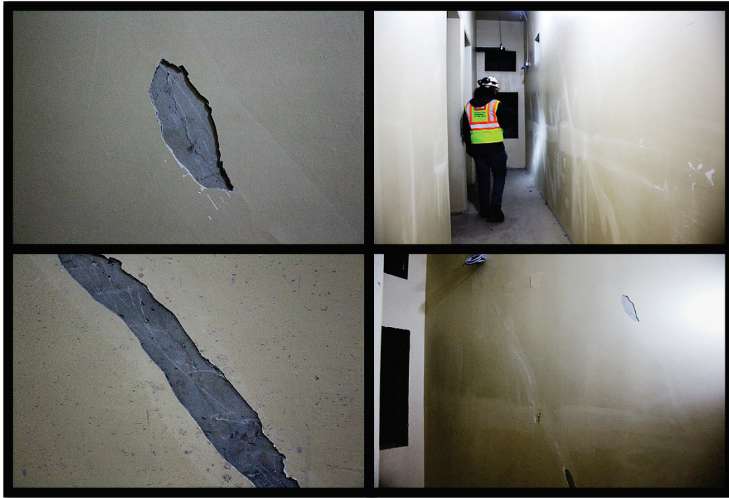
Figure B40. Diagonal cracks in basement walls of Tower 4.
