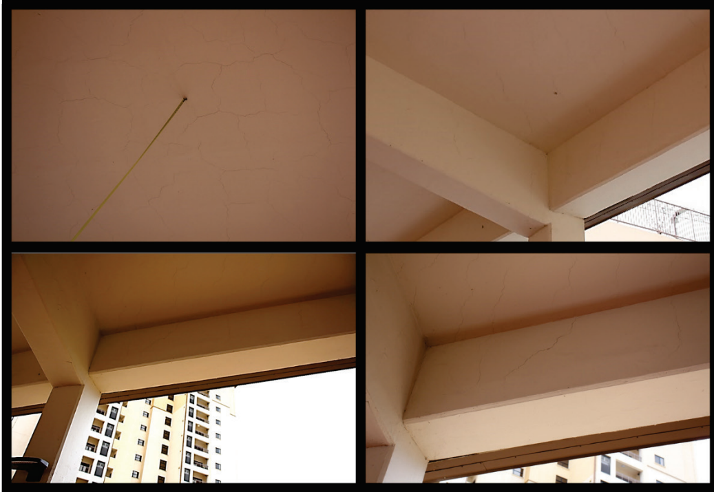
Figure B62. Multidirectional cracks in ceiling and cracks in girder of entryway of Parking Garage 2.
