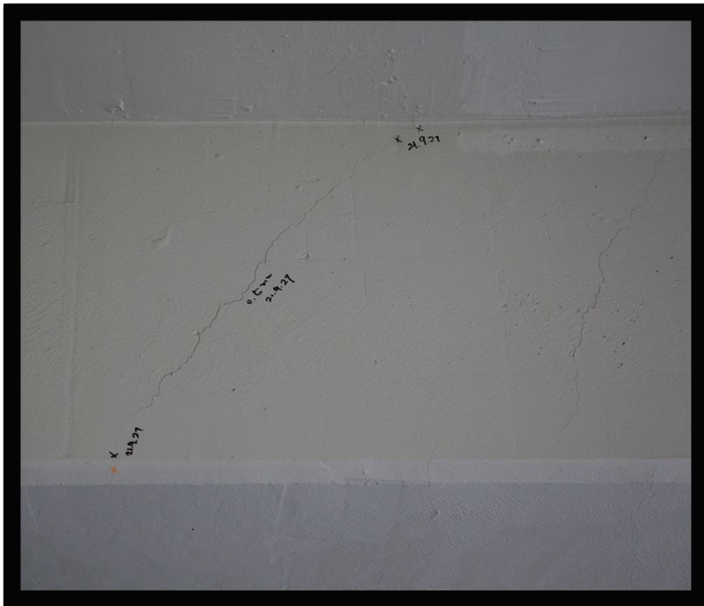
Figure 44. Typical diagonal crack in beam showing decrease in crack width at bottom and top of beam.
