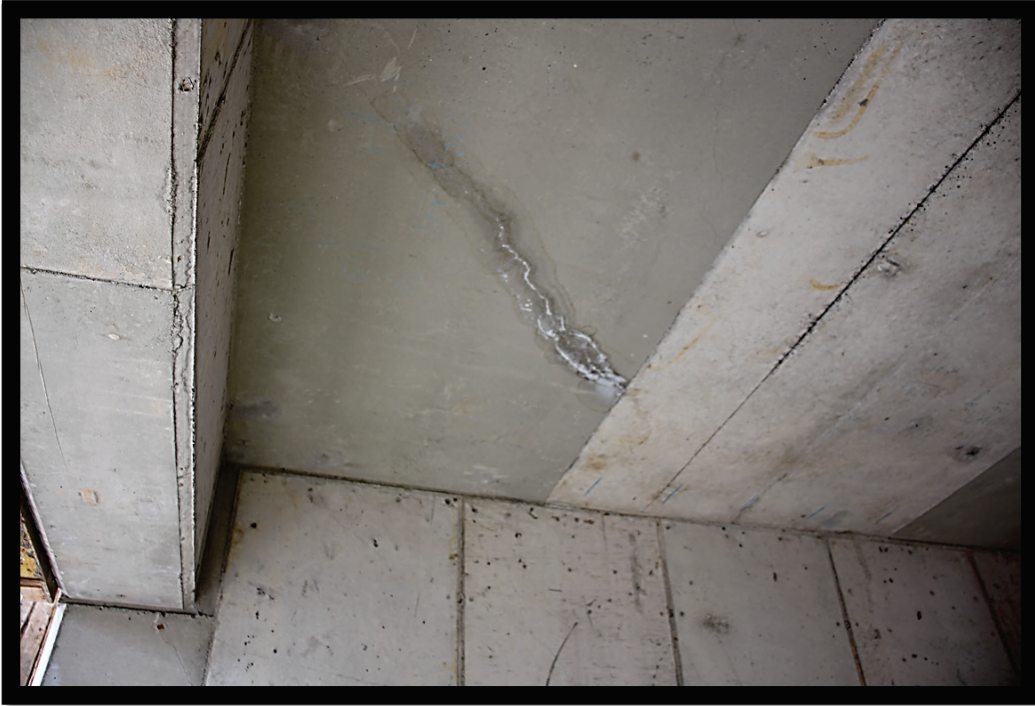
Figure 56. Crack in slab of Parking Garage 4 showing staining at location of water ingress.
