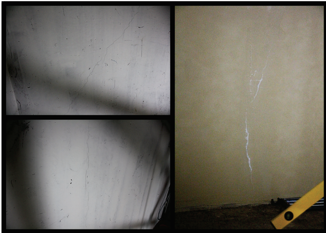
Figure B41. Cracks in walls of Tower 4.
