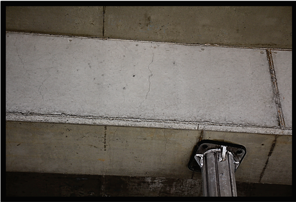
Figure 57. Vertical crack in beam immediately adjacent to shoring. This shoring was in place continuously since concrete was cast.
