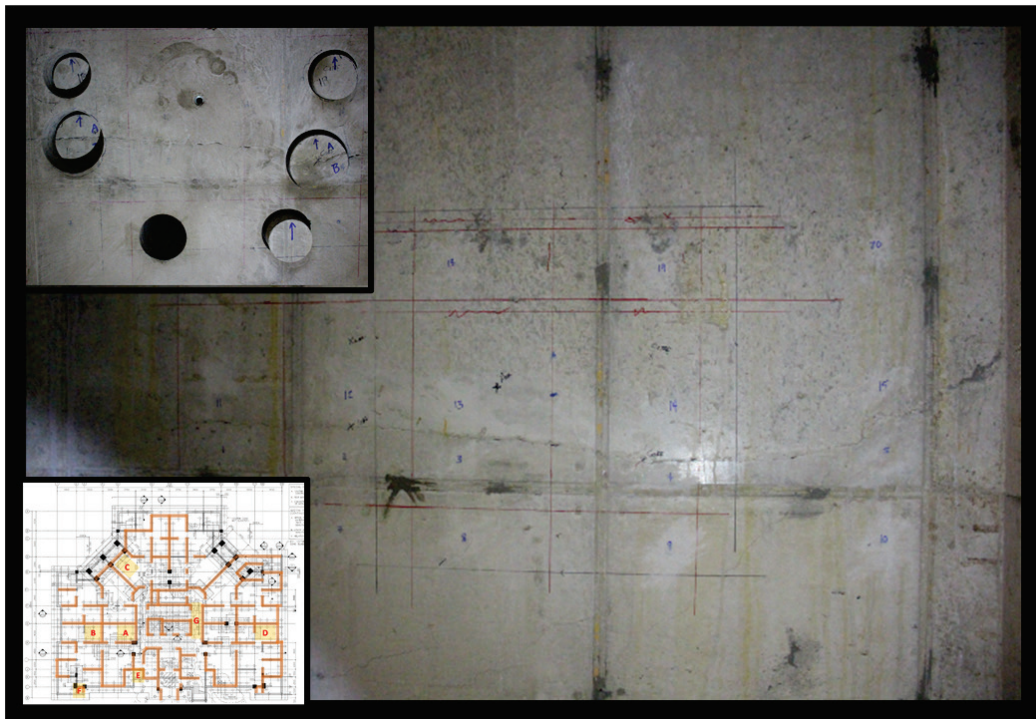
Figure D4. Prepared and cored (upper left insert) area of wall containing a cold joint in Tower 1. Red lines indicate locations of internal reinforcement.
