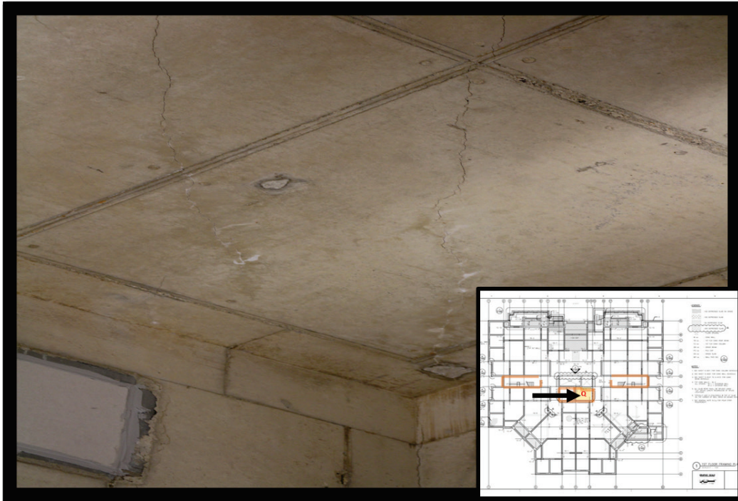
Figure 17. Typical observed overhead (ceiling) slab cracks within the Tower 2 (Section Q of the 1st Floor floorplan insert).
