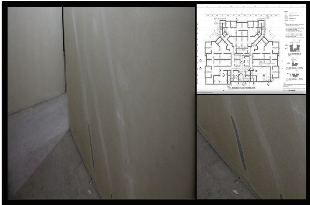
Figure 27. Typical diagonal cracking observed in the basement of Tower 4 (floorplan insert). The cracking was covered post placement but before visual inspections (insert shows the inspected crack on bare concrete without patch).
