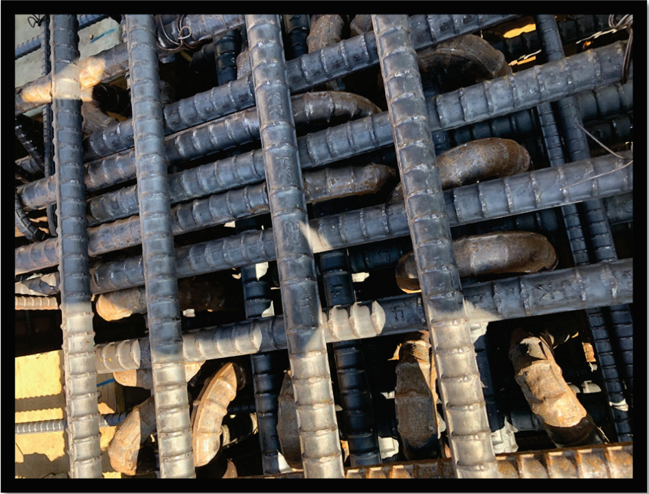
Figure 39. Rebar congestion at intersection between beams and column in Parking Garage 4.
