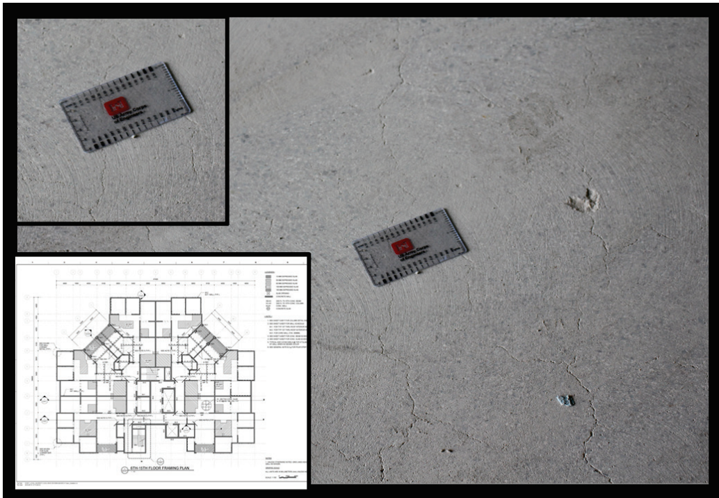
Figure 30. Observed slab cracking in Tower 4 (floorplan insert). The crack widths were less than 0.15 mm (crack gauge insert).
