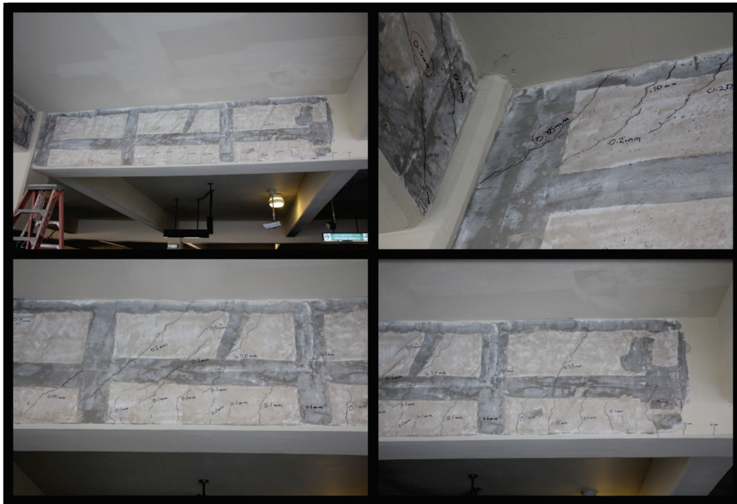
Figure B61. Mapped cracks in bare concrete of girder along column line E in Parking Garage 1.
