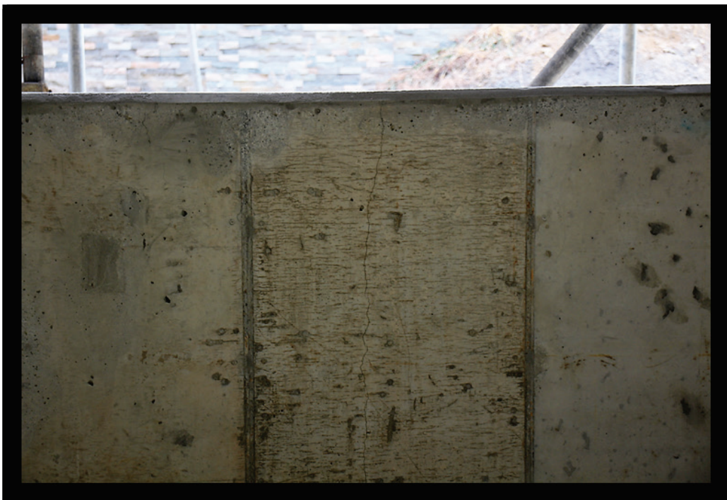
Figure B71. Vertical crack in wall in Parking Garage 4.
