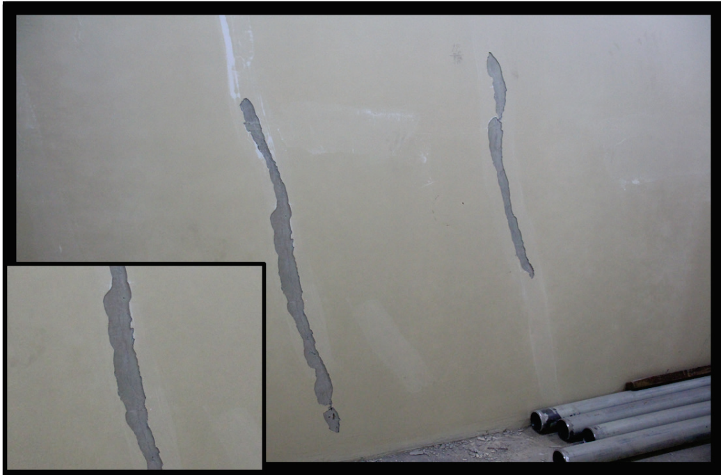
Figure 28. Vertical cracking observed in the basement of Tower 4 (floorplan insert). The cracking was covered post placement but before visual inspections (insert shows observable crack after patch/paint removed).
