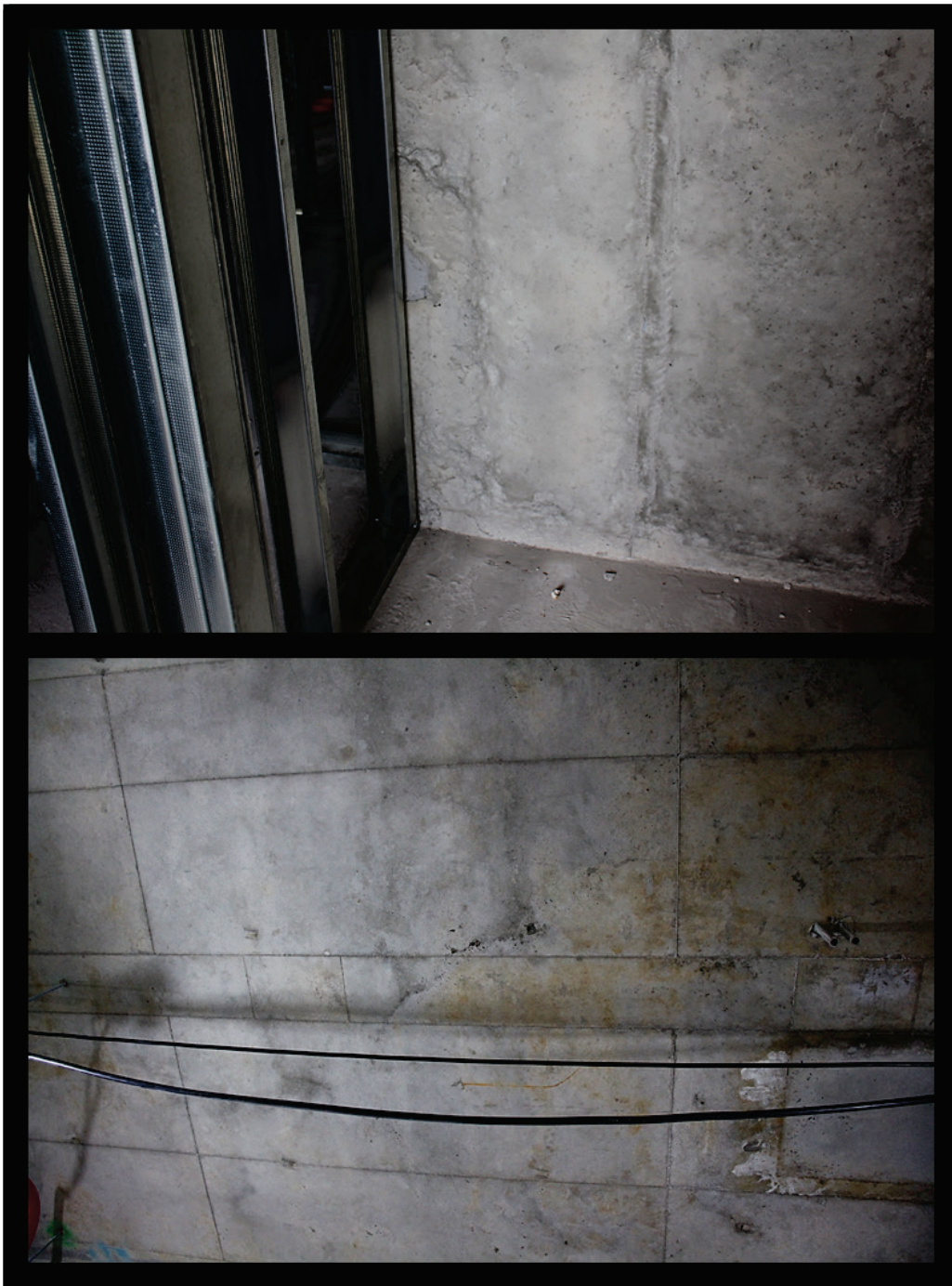
Figure B44. Nonuniformity (top) and staining (bottom) of concrete in Tower 4.
