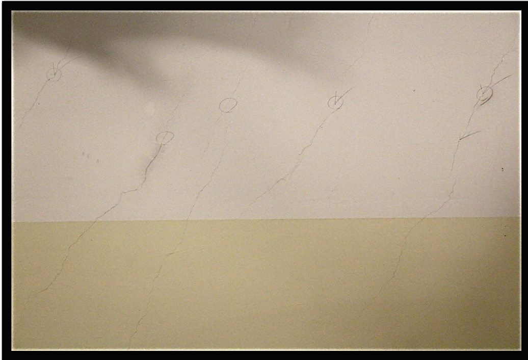
Figure 47. Diagonal cracks in first floor (basement) of Parking Garage 1.
