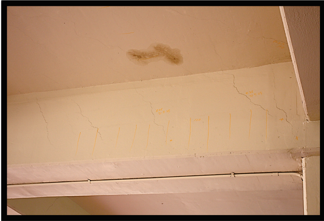
Figure 49. Typical diagonal cracking in girder of Parking Garage 2. Note the staining near a crack on the ceiling indicating water coming through from the upper floor.
