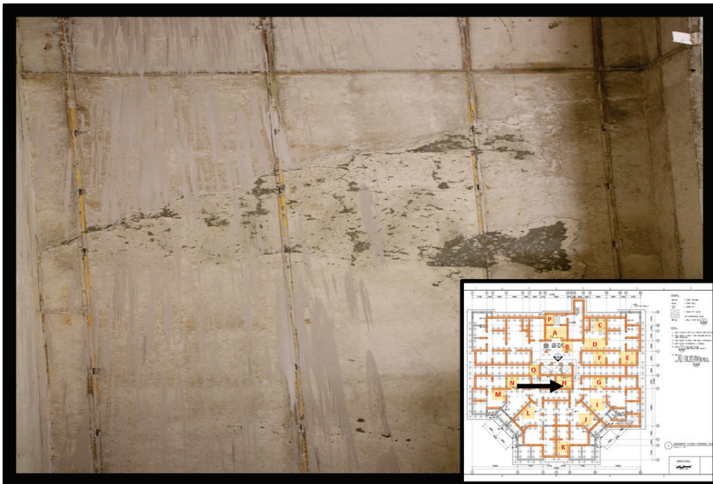
Figure 18. Observed cold joints within the Tower 2 elevator shaft area (Section H of the floorplan insert). These cold joints were observed on bare concrete and were typical in the elevator shaft areas in the upper floors.
