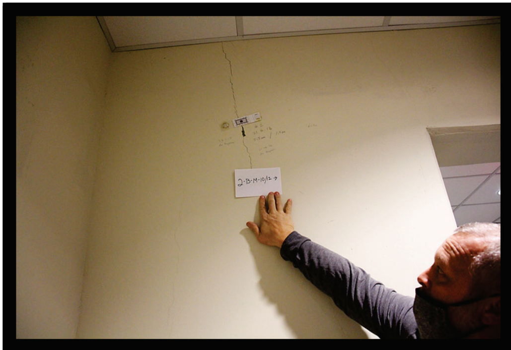
Figure B13. Wall crack with gauge in Tower 2 basement.
