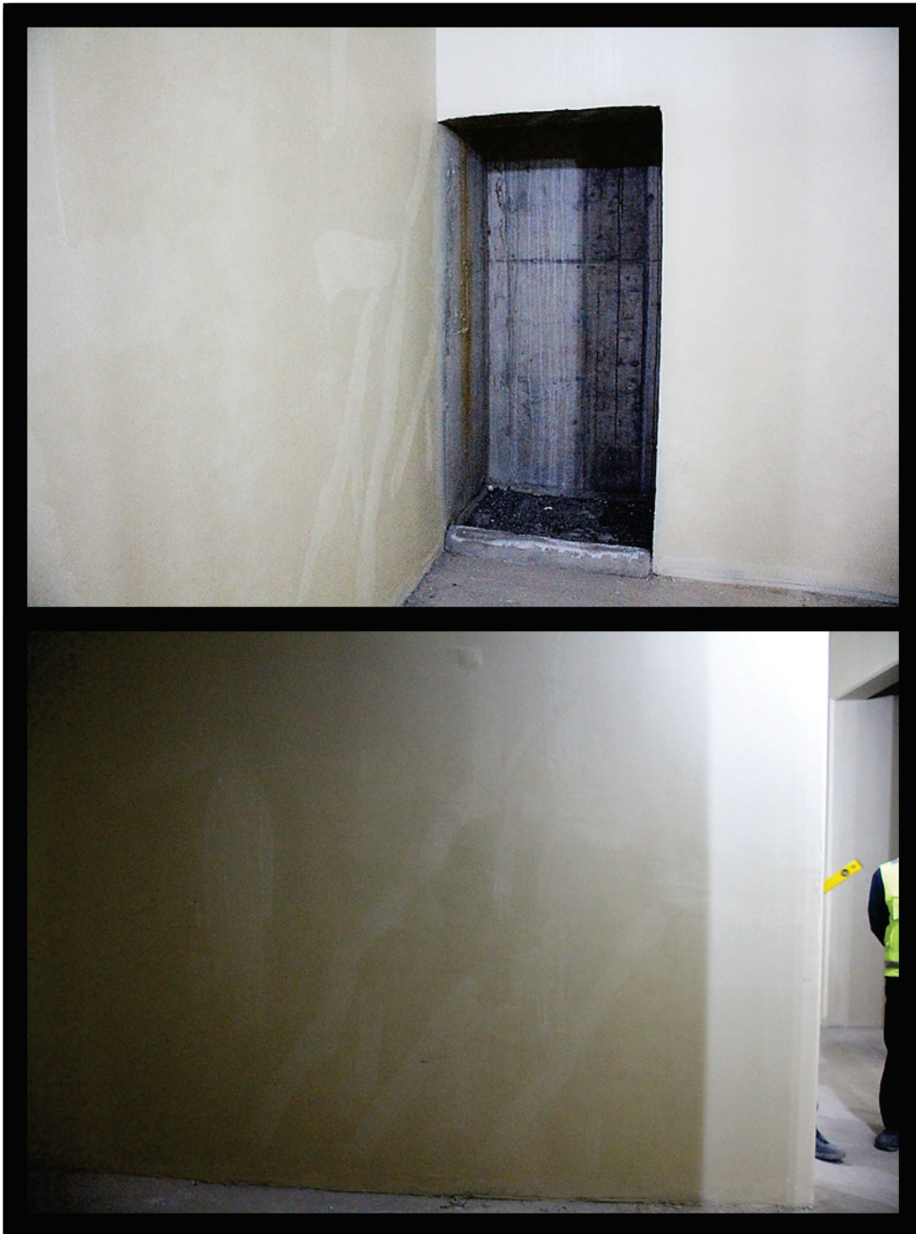
Figure B39. Diagonal cracks in basement walls of Tower 4.
