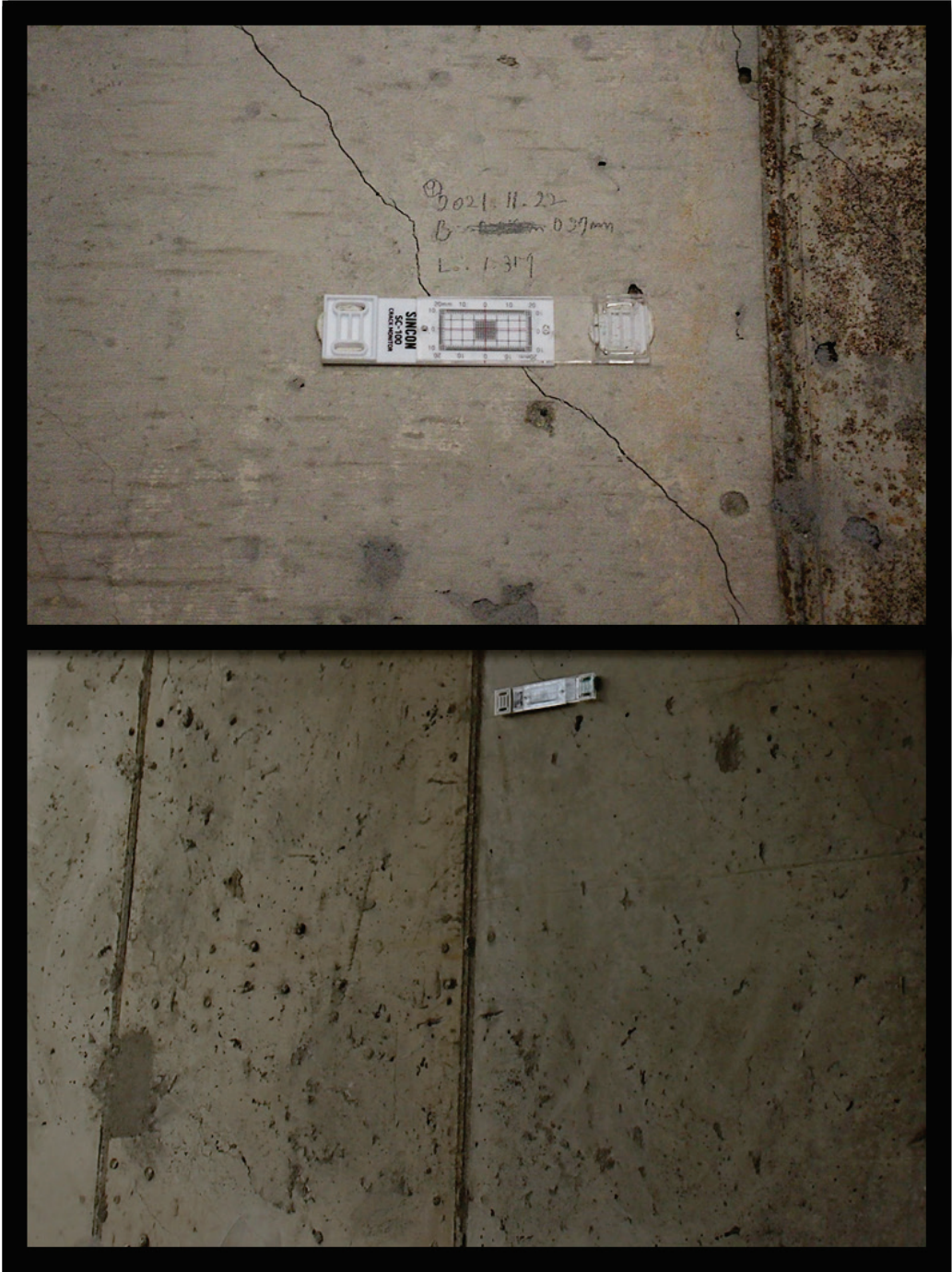
Figure B69. Cracks with gauges and bugholes in walls in Parking Garage 4.
