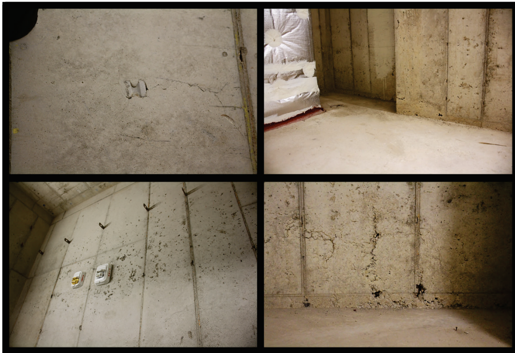
Figure B24. Embedded rebar support (top left) and honeycombing and poor consolidation in shafts behind elevators in Tower 2.
