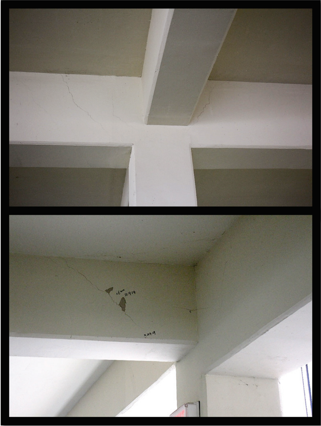
Figure B63. Diagonal cracks in girders and beams in Parking Garage 2.
