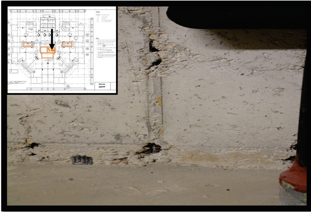
Figure 20. Honeycombing within Tower 2 (Section TAA of the 12 th Floor floorplan insert). The honeycombing varied in severity but was typically located in areas of high rebar congestion and was often near cold joints.
