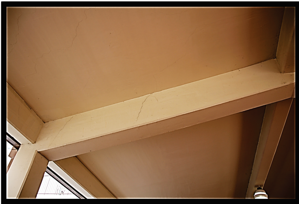
Figure 48. Crack in roof beam over Parking Garage 1 ramp. Crack width was approximately 1.2 mm.
