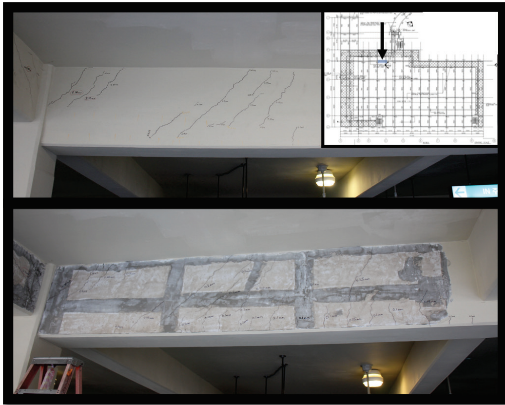
Figure 42. Comparison of crack pattern and width above and below coating in Garage 1. The crack patterns did not change when the surface coating was removed, and the widths were all within 0.05 mm of those measured on top of the coating.
