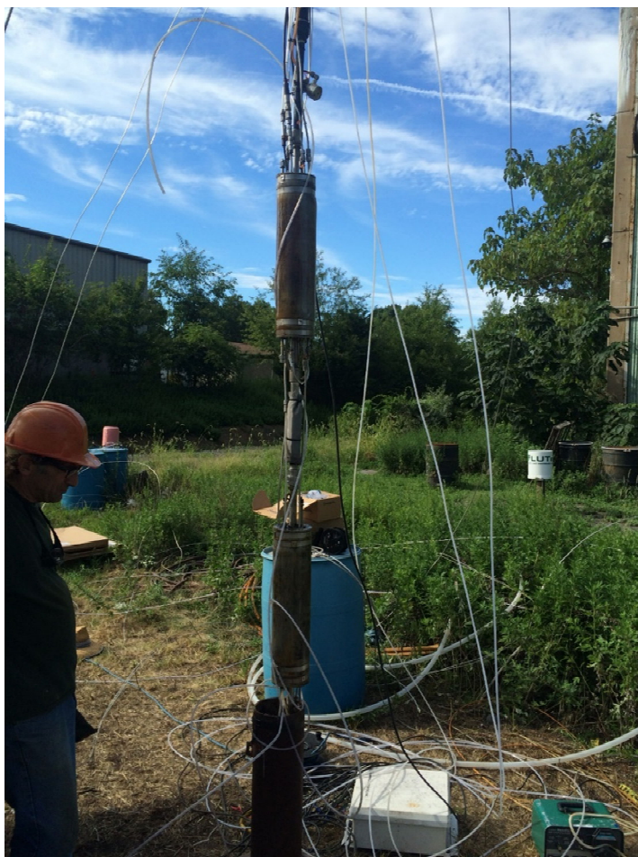
Figure ES- 2. Custom-manufactured packer system being lowered into borehole for field testing. The tool is fabricated to minimize reaction between the contaminants and test materials; all tubing is stainless steel and the packer bladders are constructed of viton. A microbial sampler (stainless-steel mesh bag containing inert sand support) is fixed in between the packers and will be exposed in the test interval.
