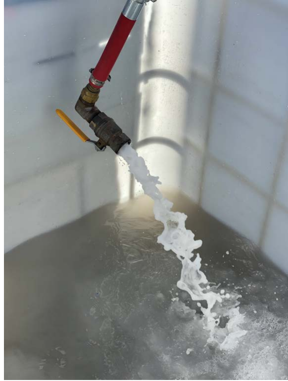
(b) Captured effluent during washout exhibiting a white color due to the cellulose.
