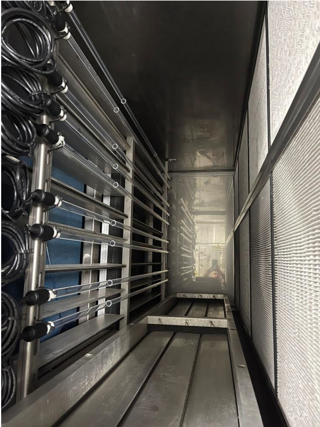
Figure 27. Main air handling unit (AHU) with Sorption wheels (energy recovery) and modulating recirculation damper-exhaust side MERV 13 pleated filters. Source: Carnival Corporation HVAC Working Group (2021).
