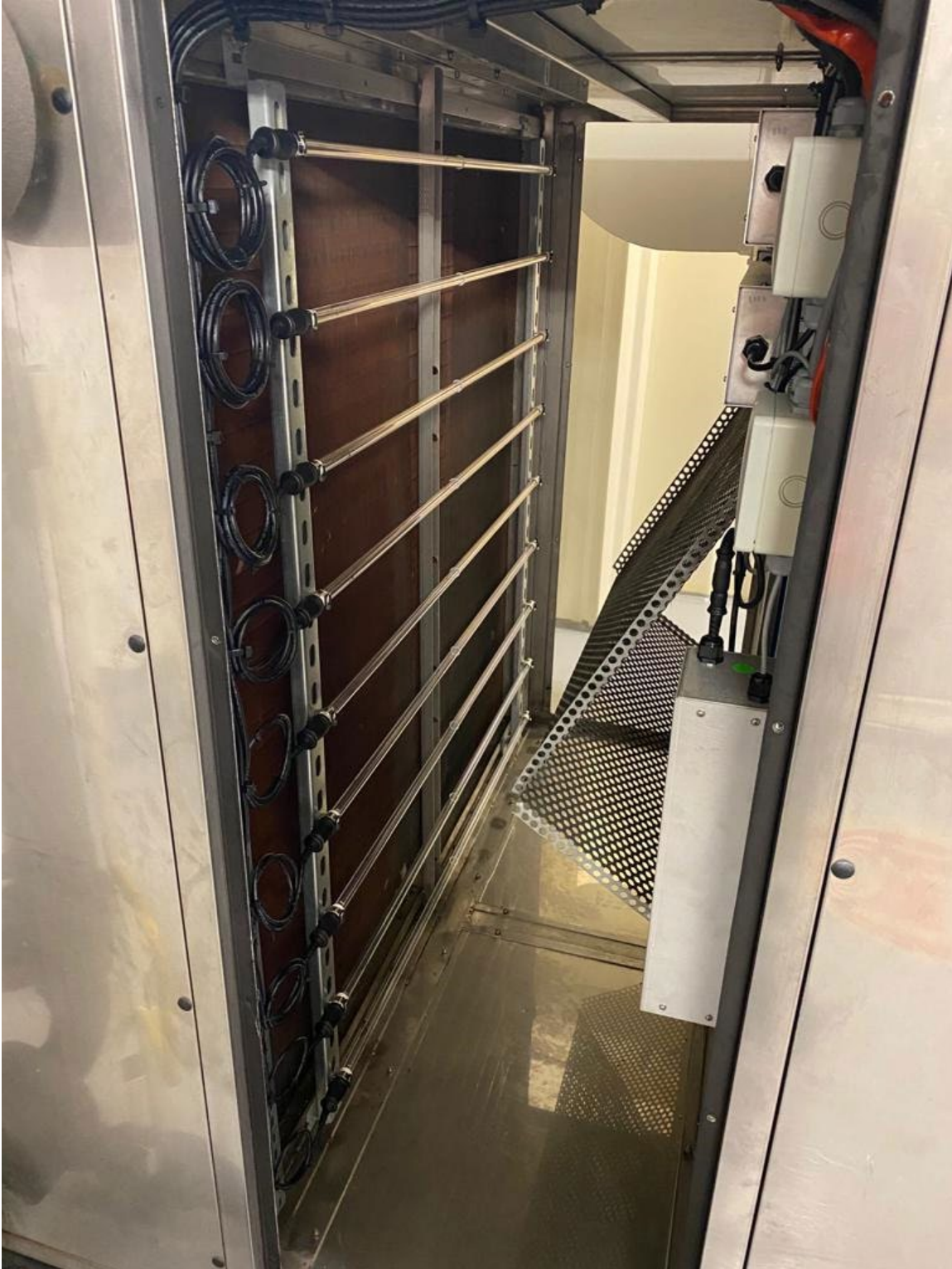
Figure 29. Main air handling unit (AHU) pushing air with UV system off. Source: Carnival Corporation HVAC Working Group (2021).
