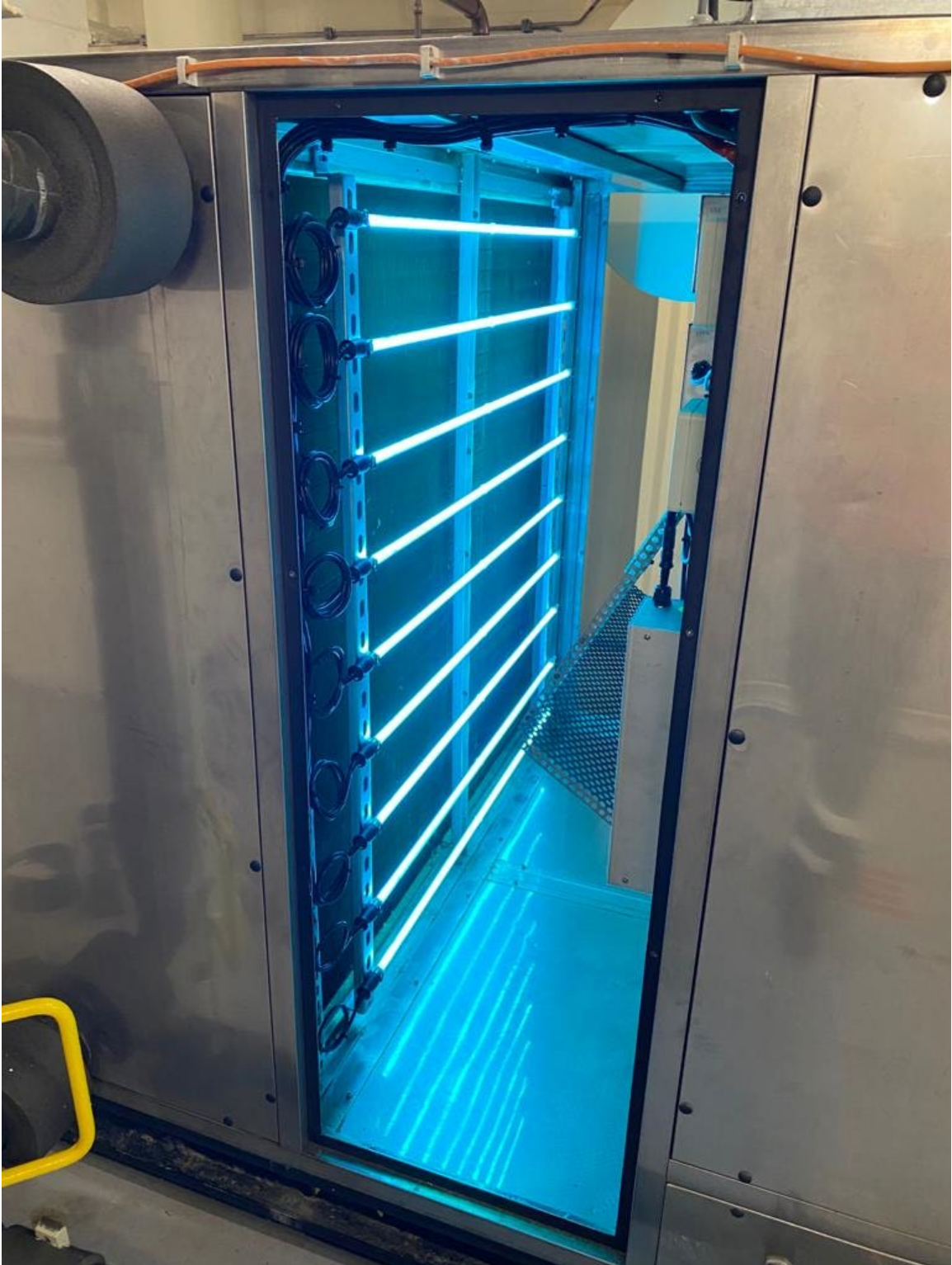
Figure 28. Main air handling unit (AHU) pushing air with UV system on. Source: Carnival Corporation HVAC Working Group (2021).
