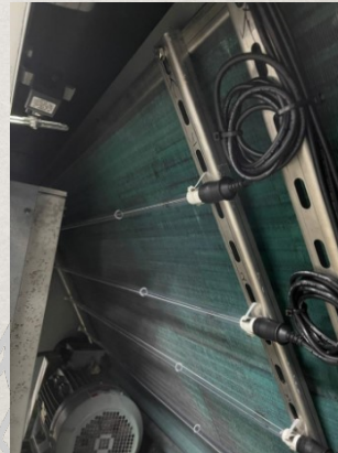
Deck-mounted public-area fan coil unit with 100% recirculation and UV off.
