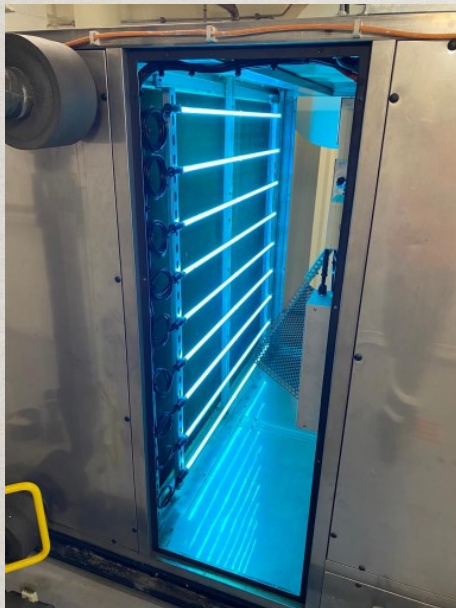
Main air handling unit (AHU) pushing air with UV system on.
