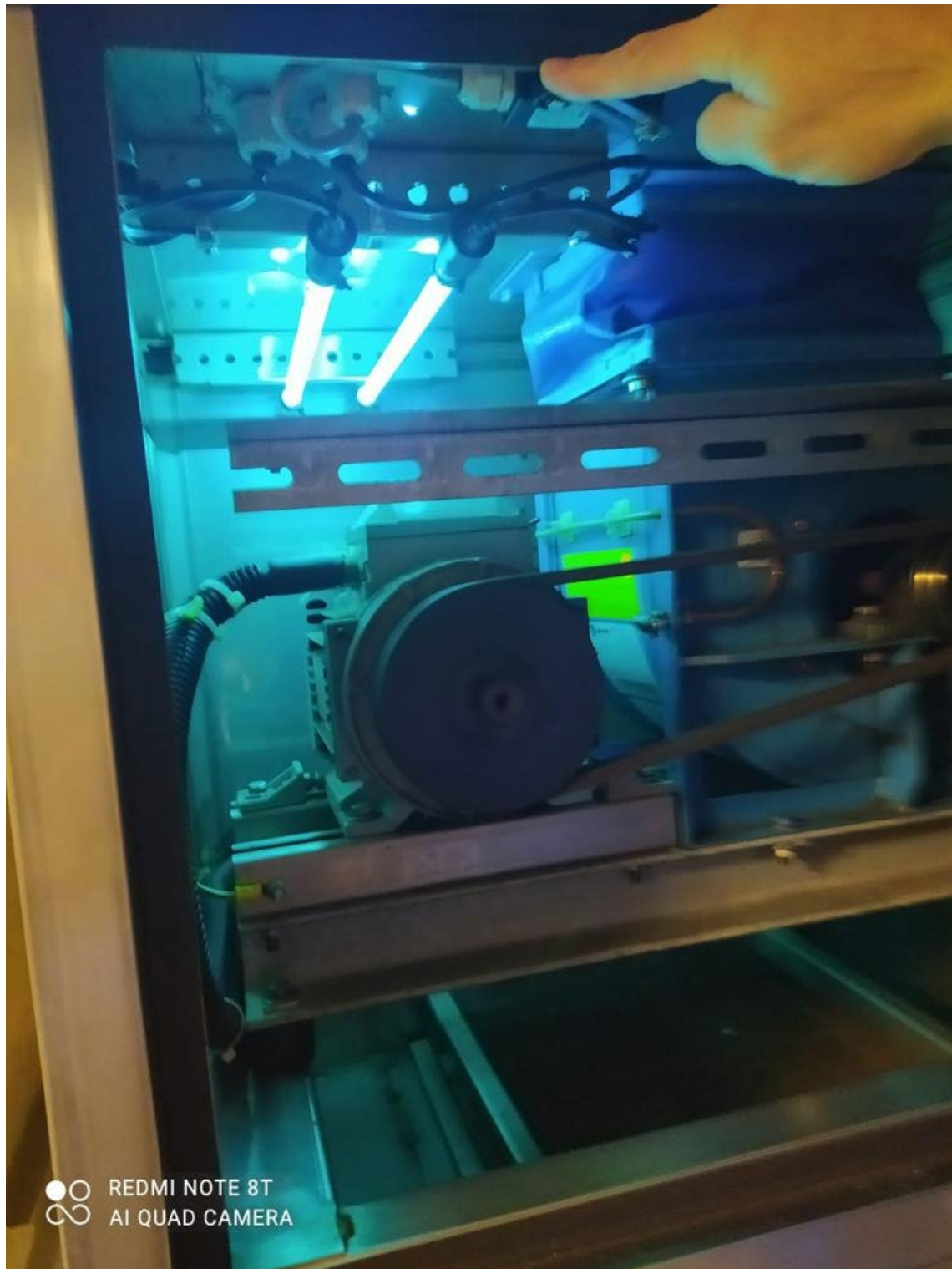
Figure 24. This image shows an operator's hand testing the limit-switch functionality, namely a safety test that the UV light stops automatically if the cover door opens. Source: Carnival Corporation HVAC Working Group (2021).
