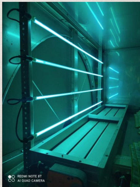
Main air handling unit (AHU) as seen from exhaust side.
