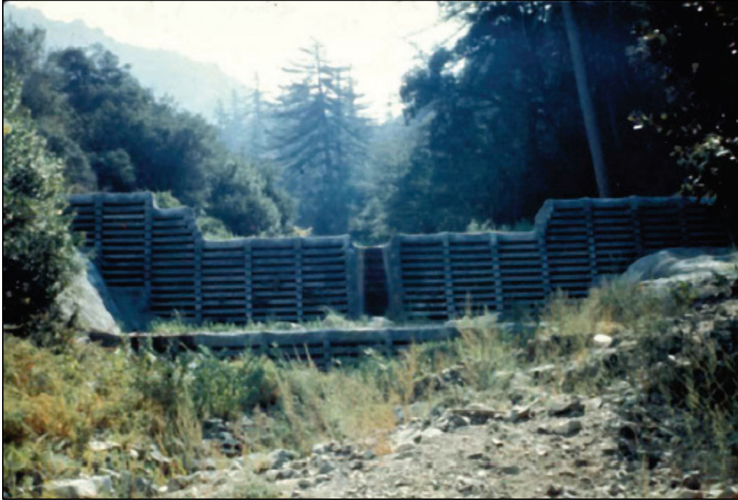
Figure 12. Debris dam made of timber (Bradley et al. 2005).
