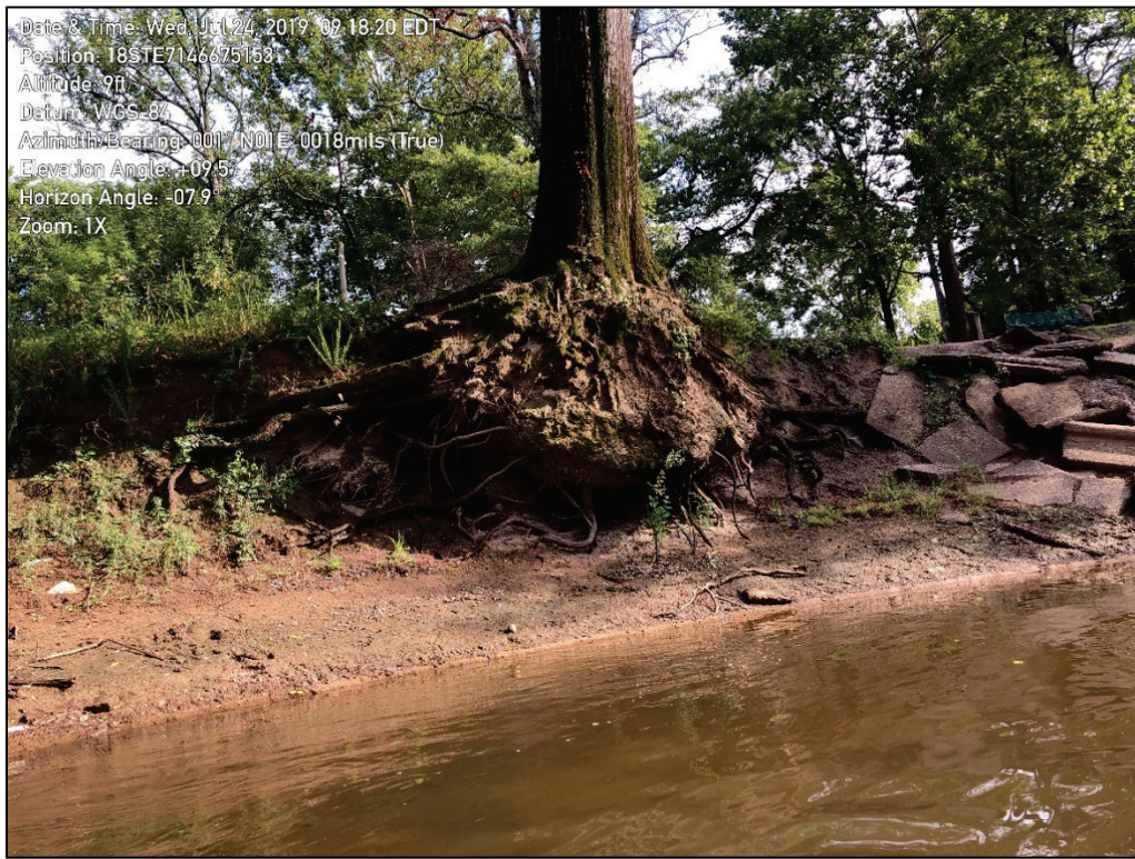
Figure A-9. A tree at risk of falling into the river as the soil around the roots erodes, seen on the Tar River near Tarboro, NC.
