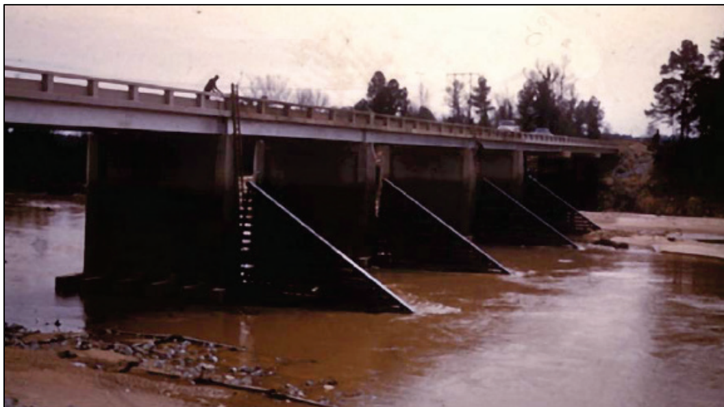
Figure 7. Debris fin deflectors diverting debris from bridge piers (Bradley et al. 2005).
