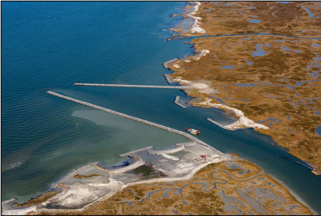
Figure 2. Aerial view of the completed jetties and sill at the Rhodes Point Navigation Project, prior to dredging and material placement in 2018 (photo credit: Coastal Design & Construction, Inc).
