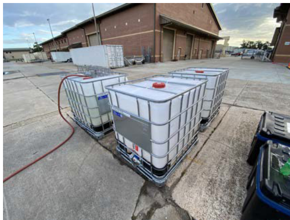
(c) Capture tanks located pier side.
