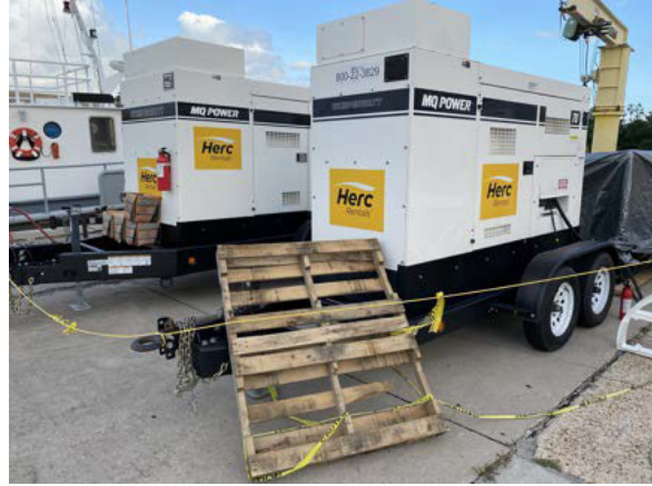
(b) Diesel-powered generators that provided electrical service to the high-pressure intensifier and other equipment.
