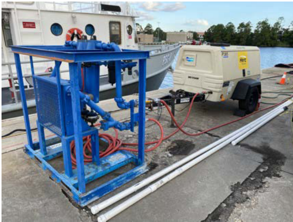
(c) Air compressor and dryer that supplied utility air to the capture pumps.
