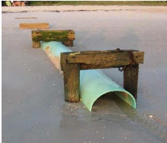
Figure 4: Inundated Stormwater Outfall at Naples Beach, FL (Naples, FL 2021)
