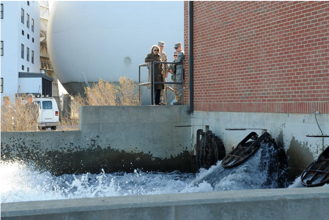
Figure 2: Demonstration of Stormwater Pump at Langley AFB (Stannard 2016)
