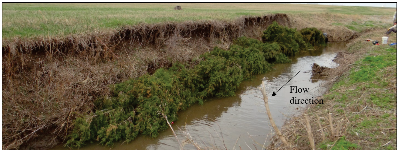
Figure 2. The completed cedar tree revetment with cedar trees anchored to the toe of the eroding bank.
