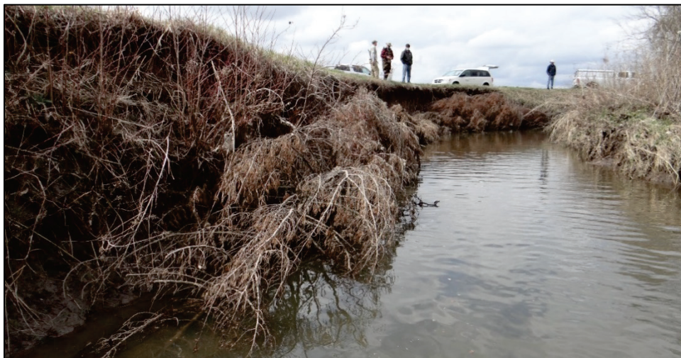
Figure 7. The upstream cedar tree revetment, installed June 2020. Photo was taken approximately 9 months post installation. Some deterioration of the trees is evident with many of the fine branches and needles missing.
