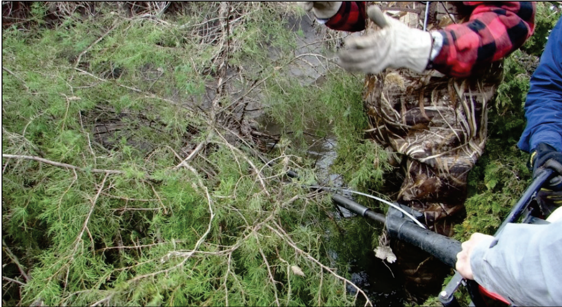
Figure 3. An anchor is driven into the bank to secure one of the cedar trees.
