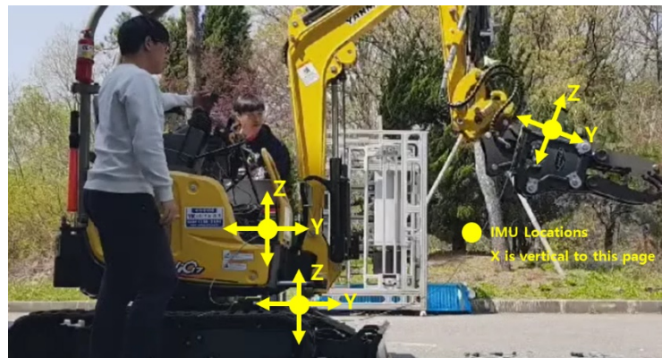
Figure 14: IMU Locations on the Remote Excavation System
