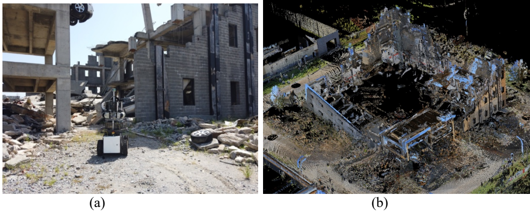
Figure 3: (a) Ground robot scanning a damaged concrete structure at Guardian Centers (b) acquired 3D point cloud of the damaged structure
