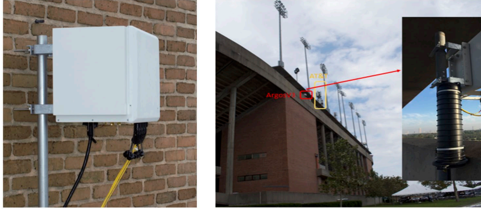
Fig. 1 RENEW base station installed at multiple locations in Rice University
