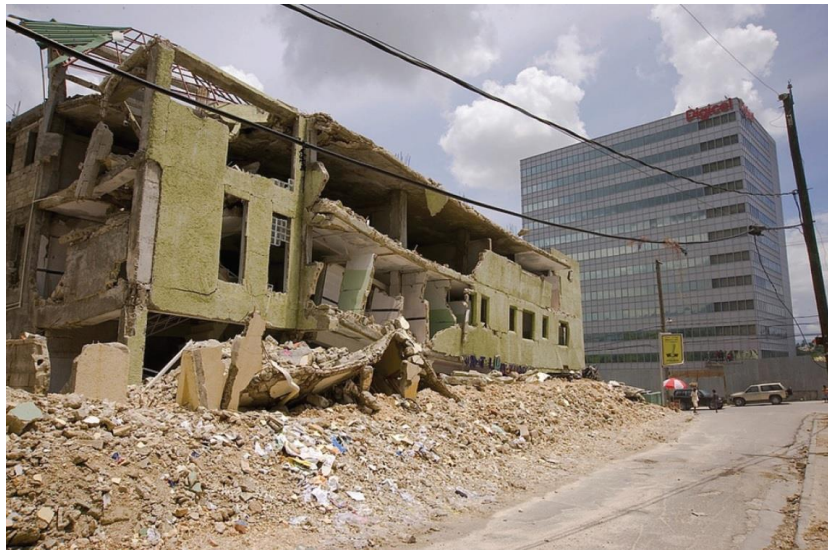
Figure 4: Digicel Building Next to Collapsed “Hopital de Turgeau” in Port-au-Prince
